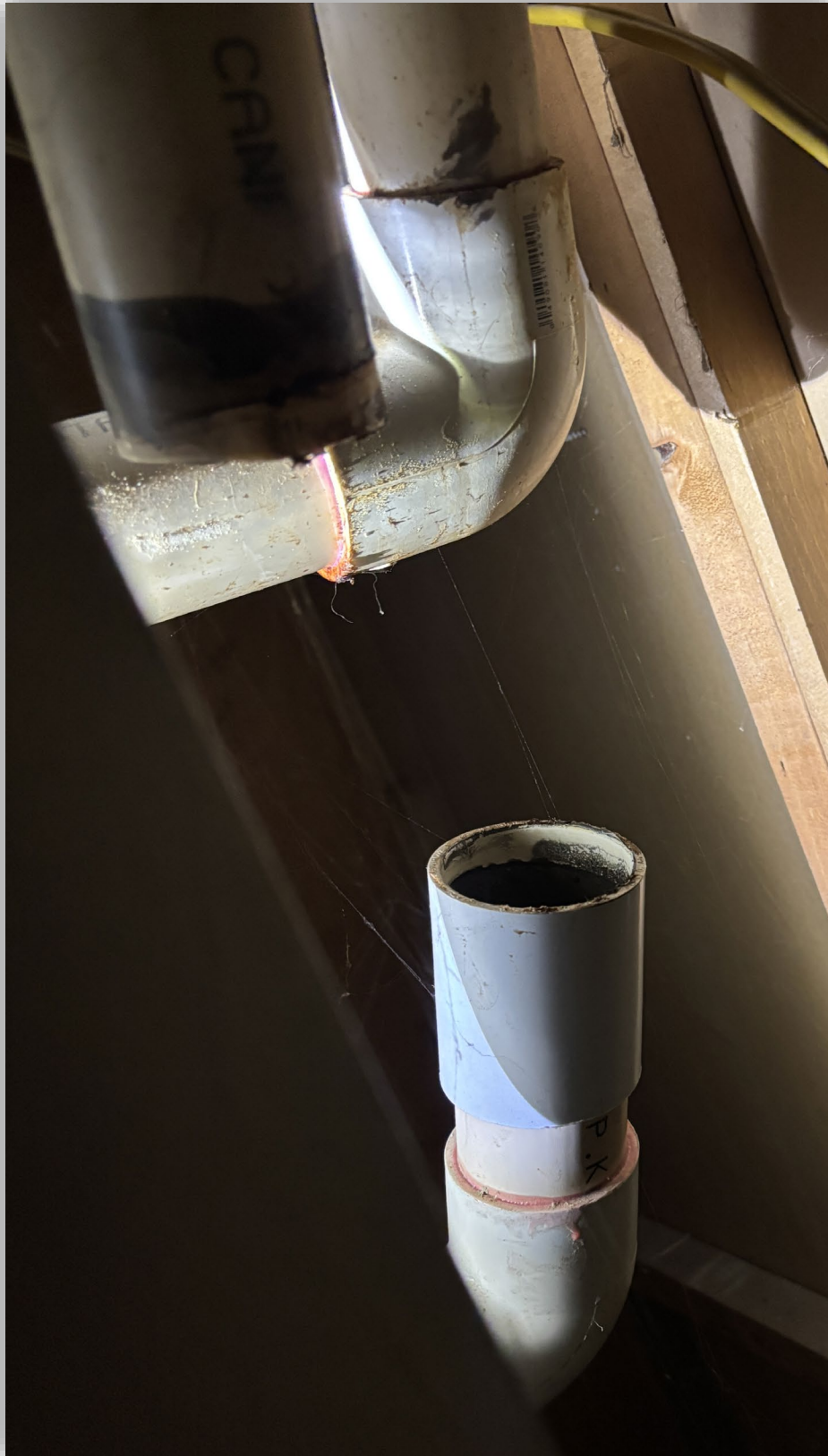
Image 7 – Disconnected flue vent pipe from other angle.
