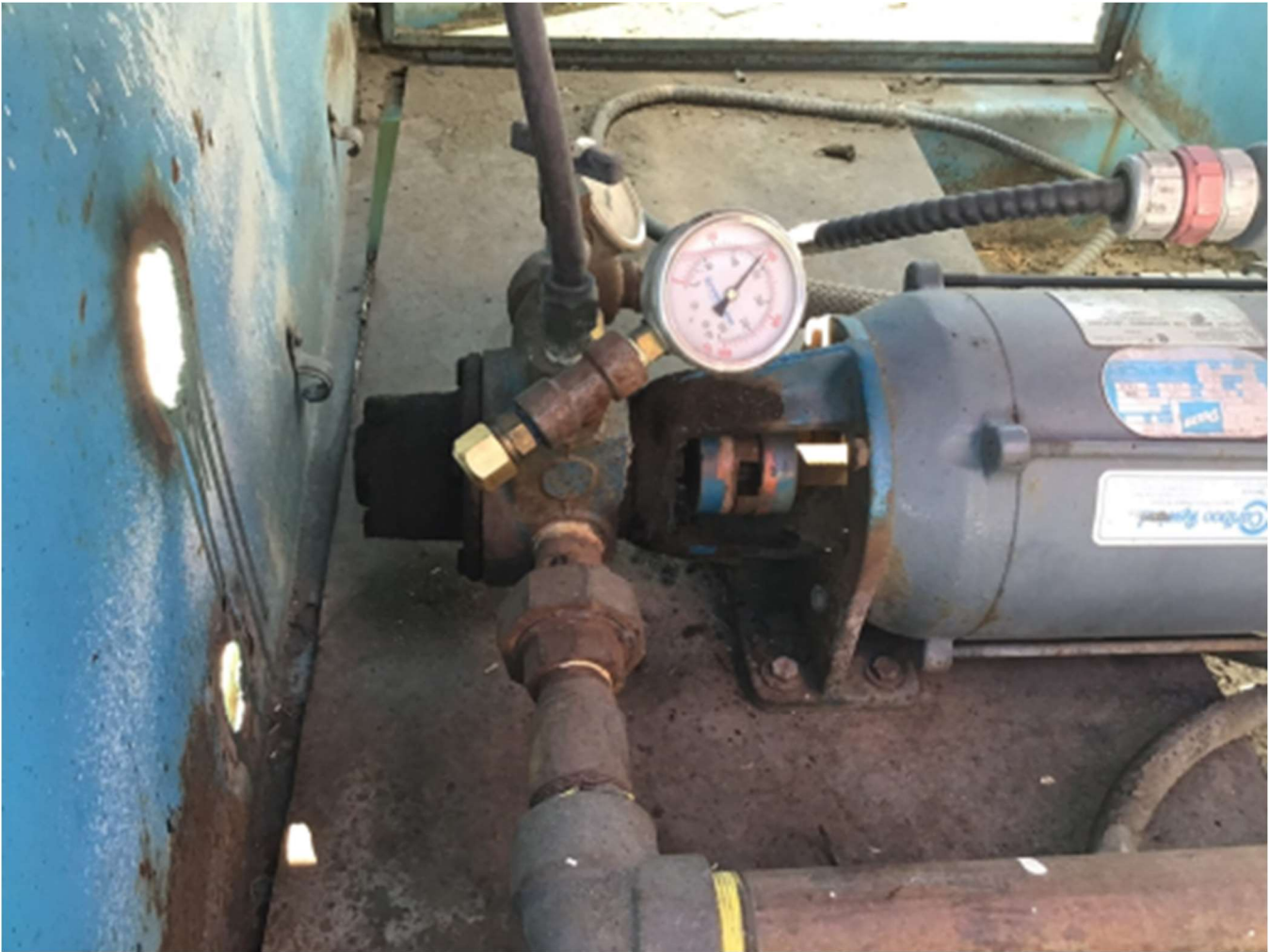
Image 1 - Discharge gauge on liquid pump, and hydrostatic relief removed
