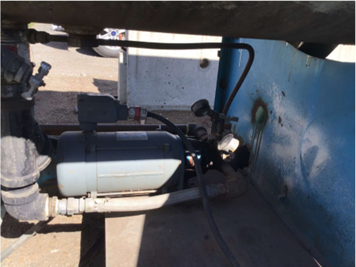
Image 2 - Pump overview and bypass
