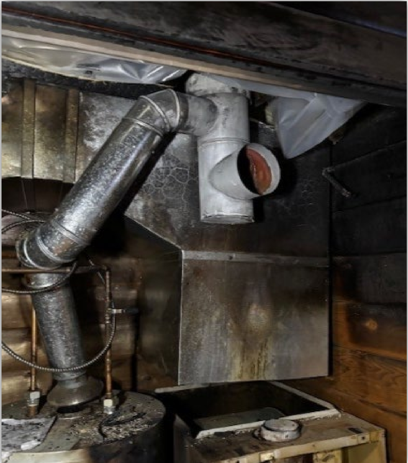
Image 2 – Close-up of damage from explosion/fire above furnace and water heater.
