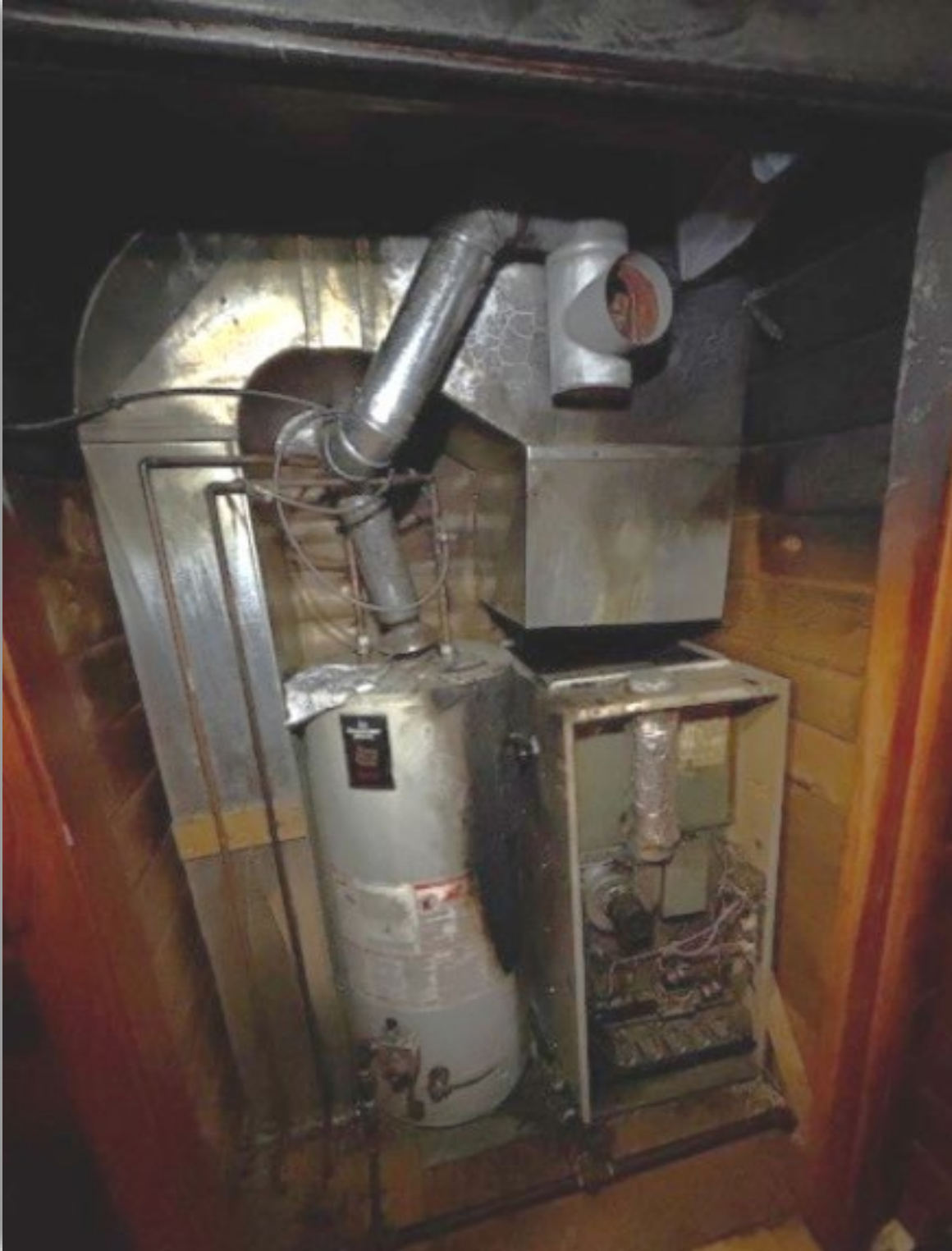
Image 1 – Furnace and water heater post-Incident in place. (Photo taken by Restoration Company.)
