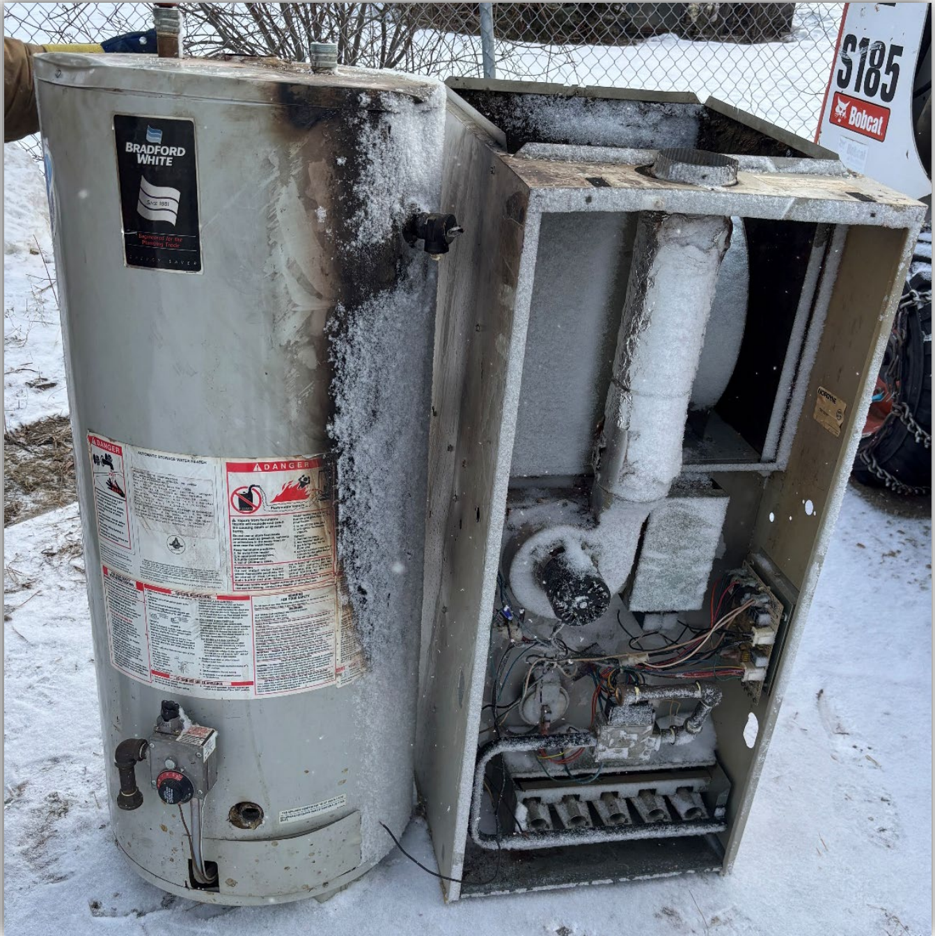
Image 4 - Furnace and water heater damaged and removed post-Incident.
