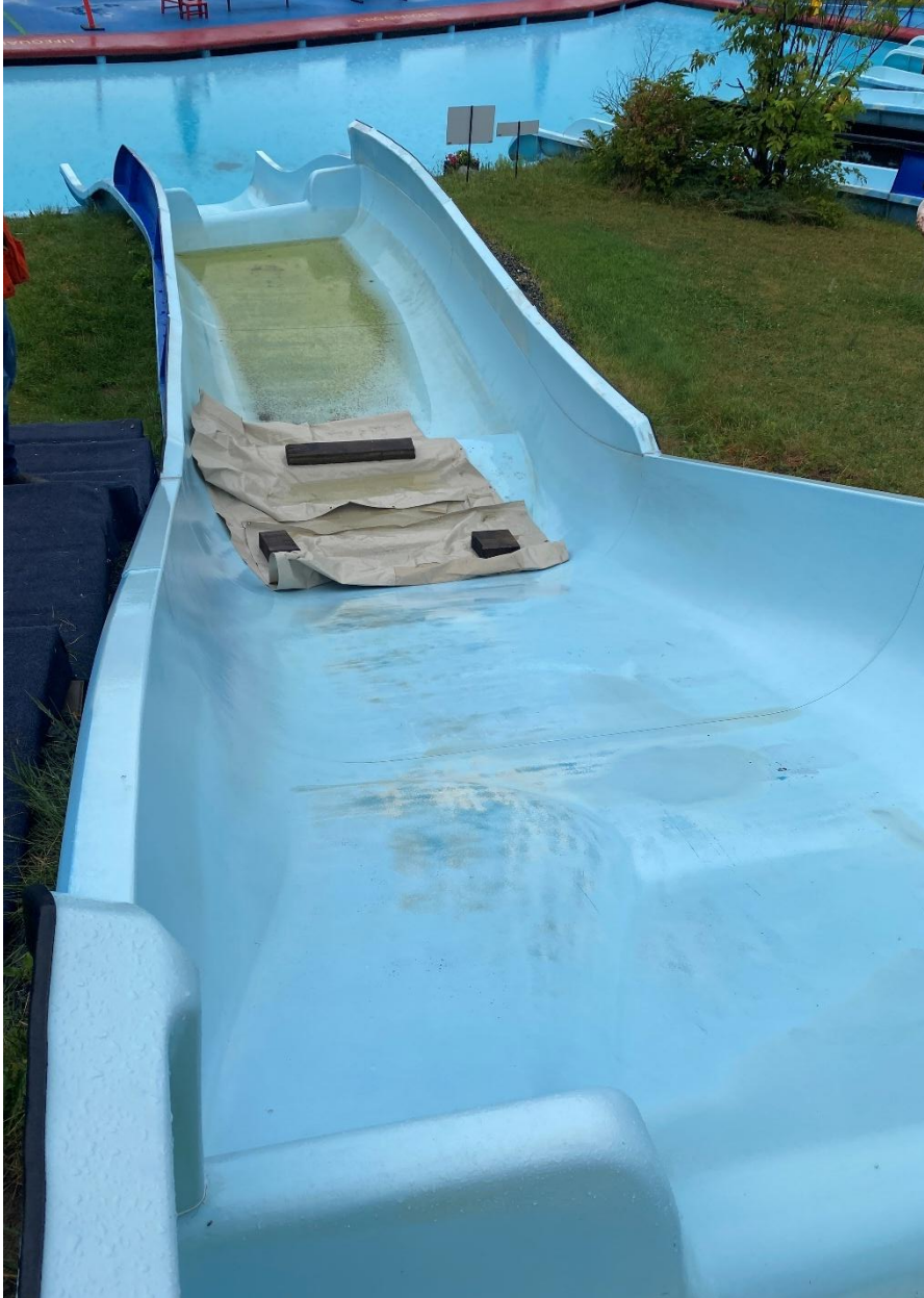
Figure 11 - Photograph taken from the position of the slide attendant who was tasked with trying to direct tubes around the downstream failure.
