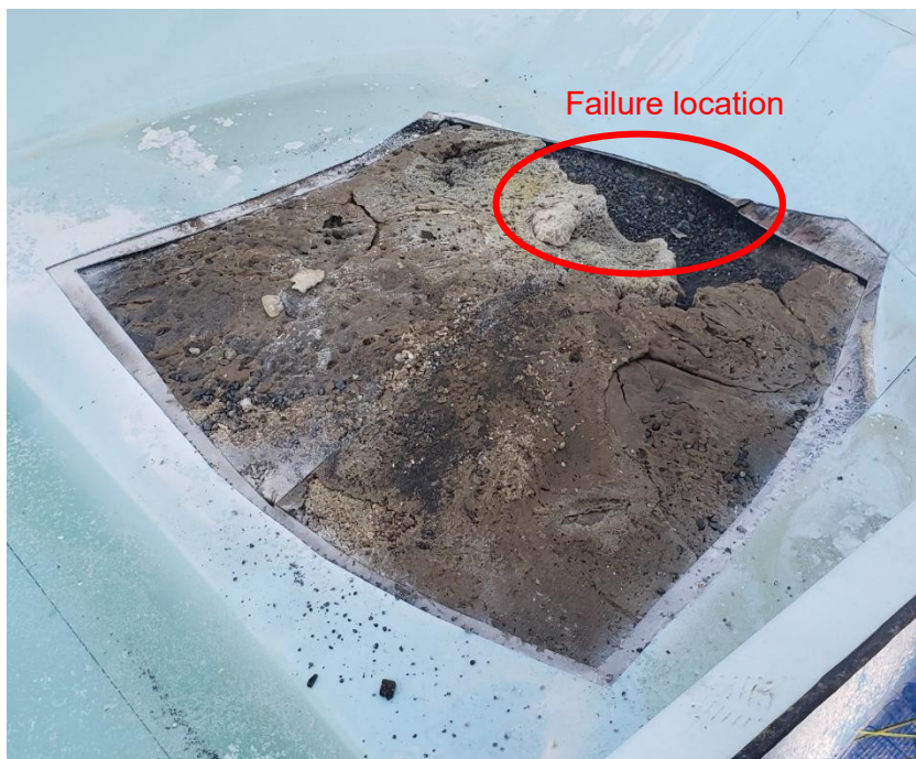
Figure 8 - Failure location after bottom layer of fibreglass was removed. A large mass of spray foam was located beneath the flume, but did not fill the area below the failure (Photograph provided by fiberglass contractor).
