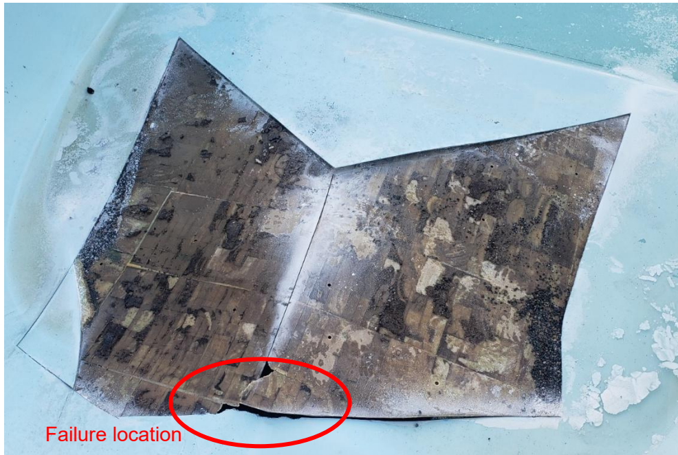
Figure 7 - Failure location, top layer of fibreglass removed. Note the wood core has completely disintegrated (Photograph provided by Fiberglass Contractor)
