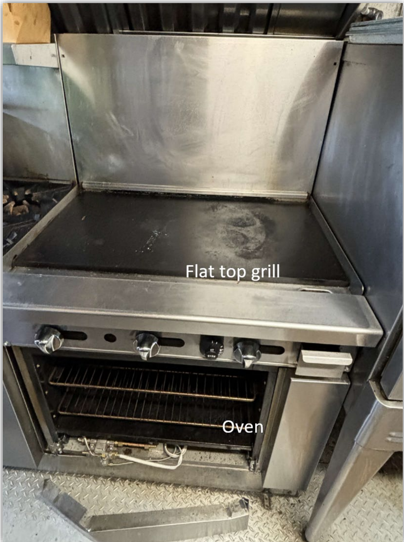
Image 2 – Upper view of cooktop and oven post explosion.
