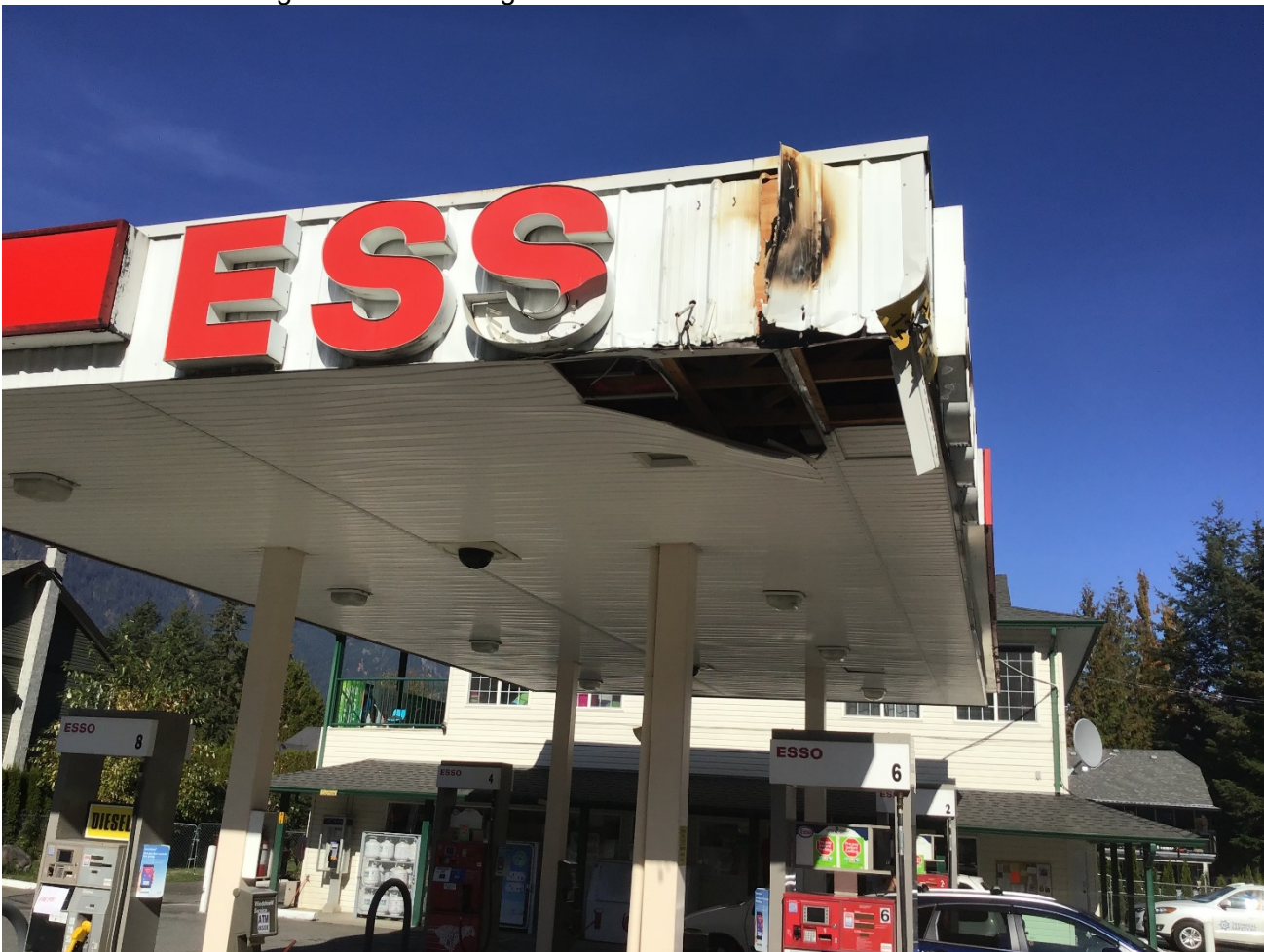
Photo of the ESSO Sign and the missing "O"
