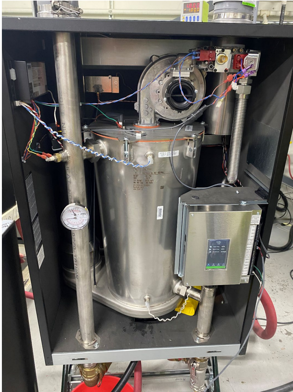
Image 4 – Boiler internals examined for damage after each test.
