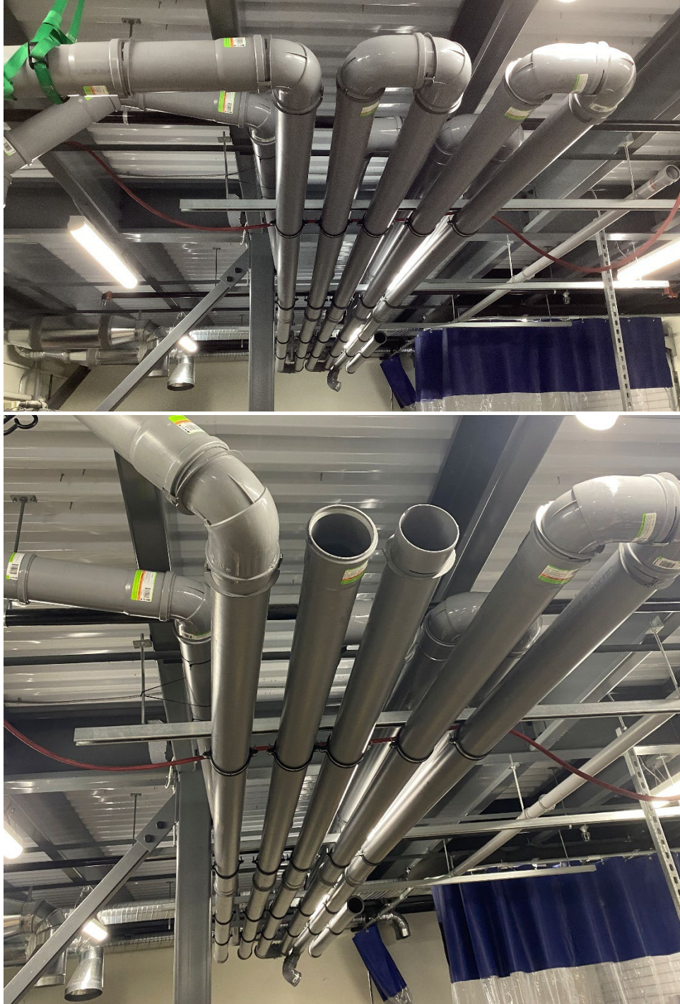
Image 8 – Boiler vent system before (top) and after (below) the 2.5-second delayed-ignition test.
