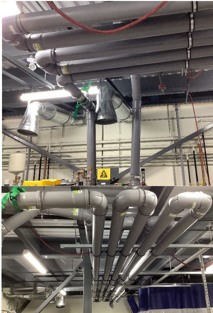
Image 1 – Venting configuration as installed.
