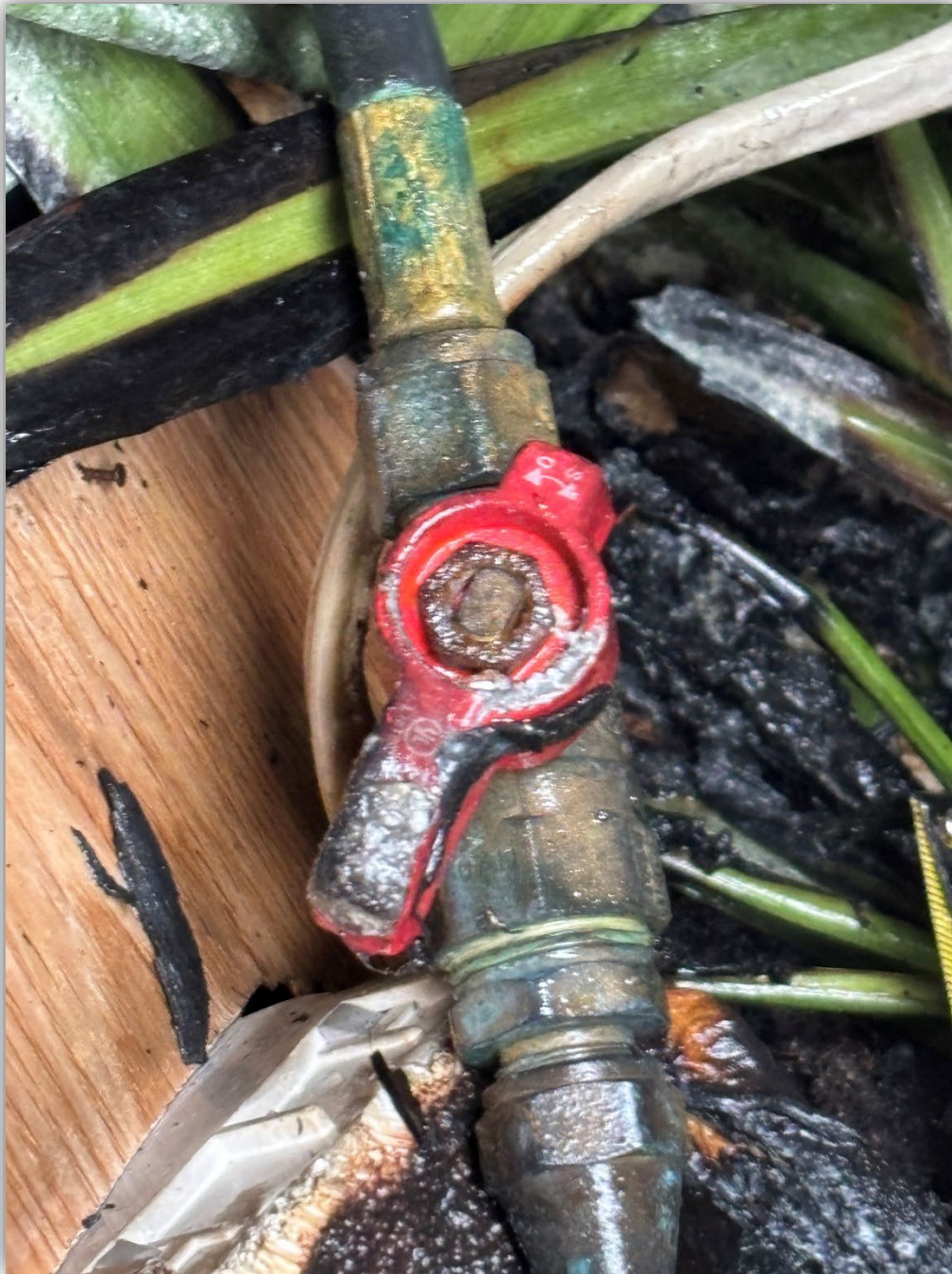
Image 9 – Close-up of the gas valve in the partially open position.
