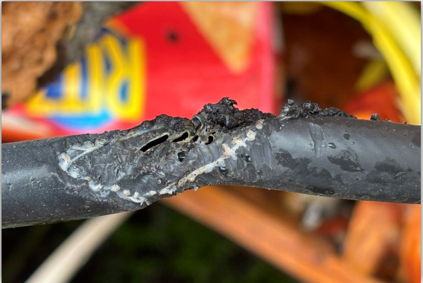
Image 7 – Close-up of rodent chew marks and holes on the rubber gas line.
