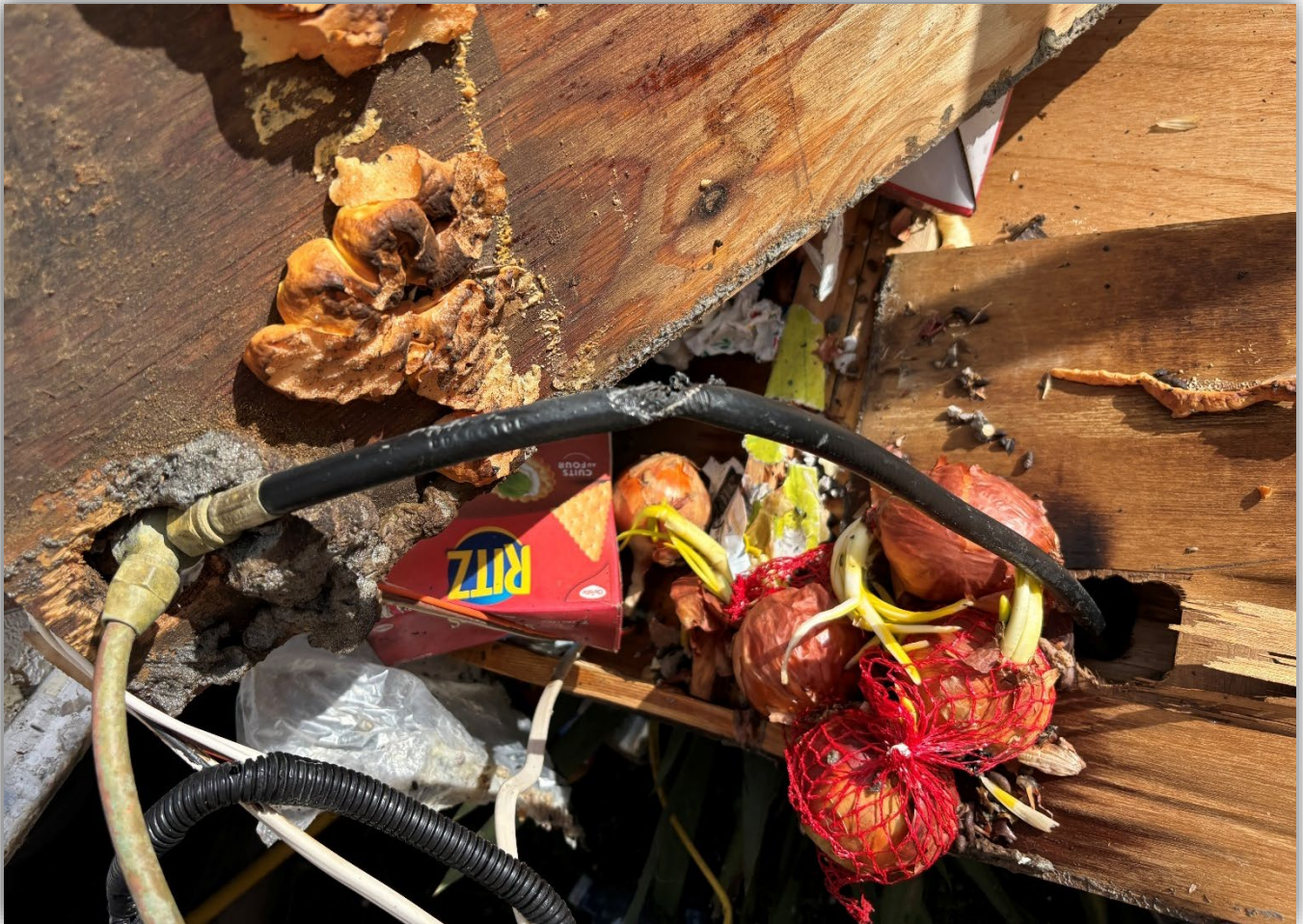
Image 6 – Copper (range) and rubber (fridge) propane gas line.
