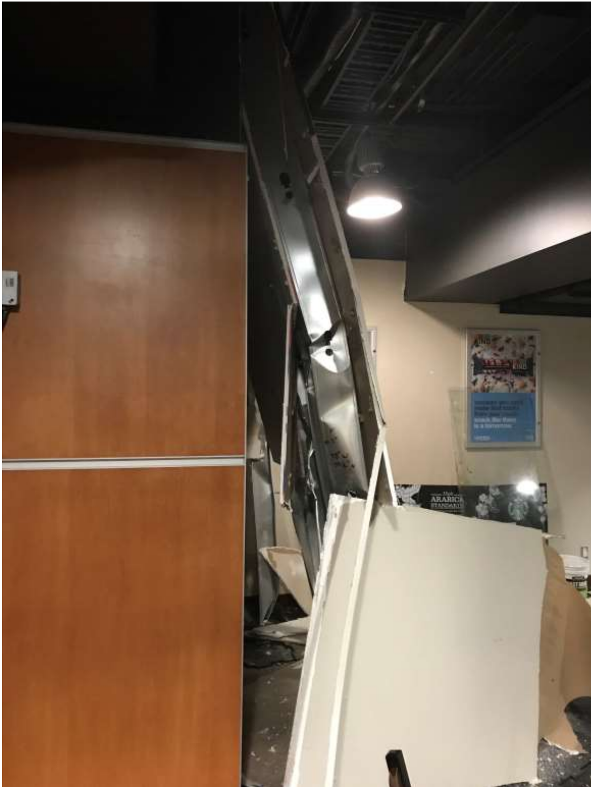
Damaged Internal Wall Side View
