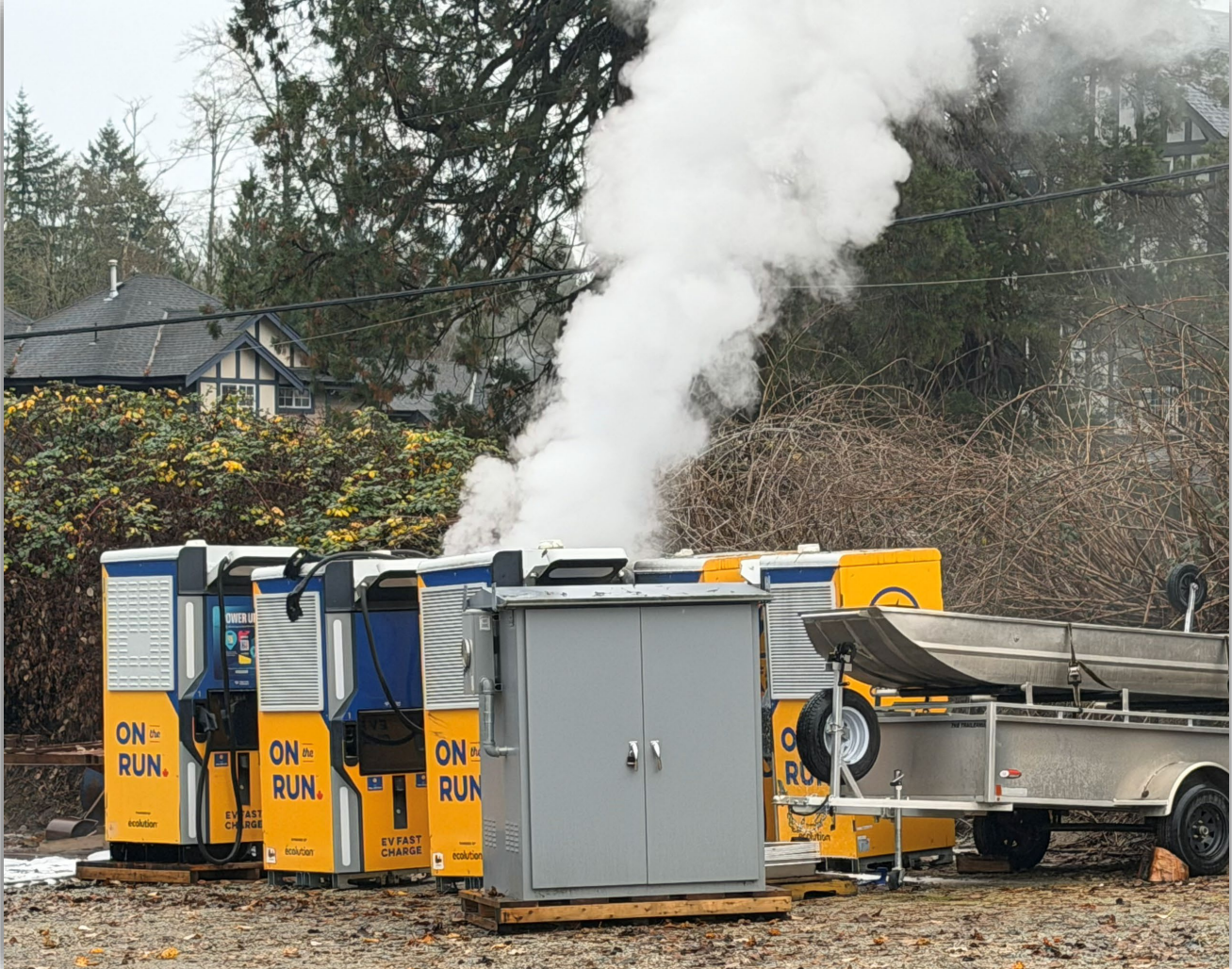
Image 2 – EV charger lithium-ion battery off gassing after flame extinguished by the fire department.
