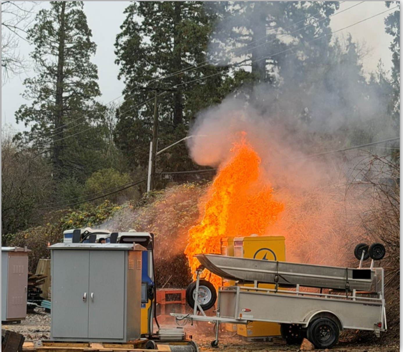
Image 1 – EV Charger on fire surrounded by other chargers in a storage yard.
