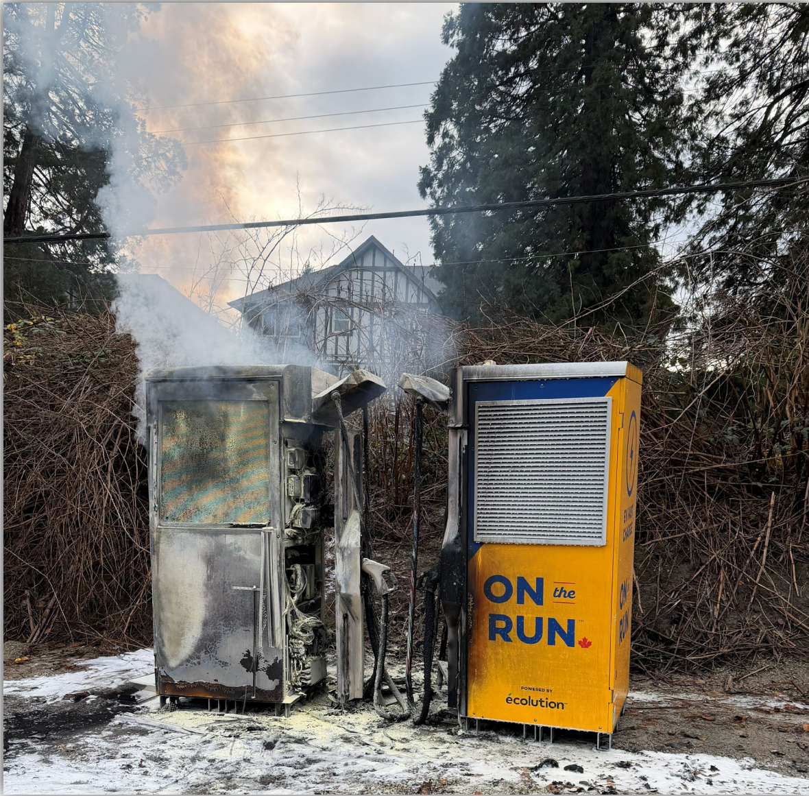
Image 3 – EV charger destroyed by fire next to another charger damaged by the fire.
