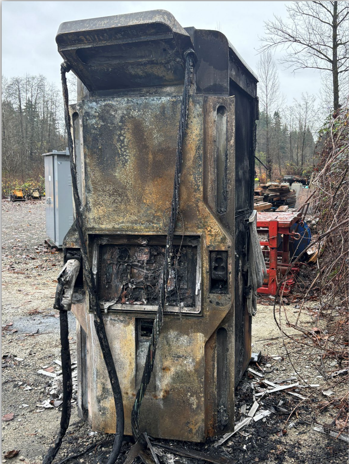
Image 4 – Damaged EV charger after fire extinguished.
