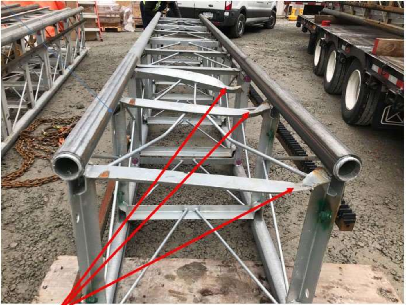
Damaged Tower Section
