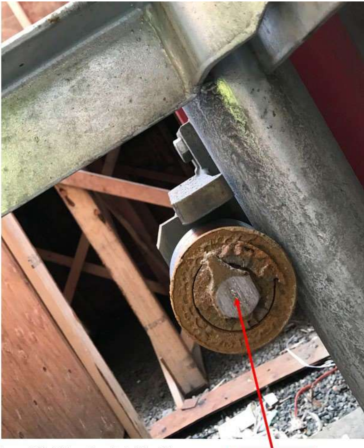
Lower Guide Roller – Opposite Building Side
