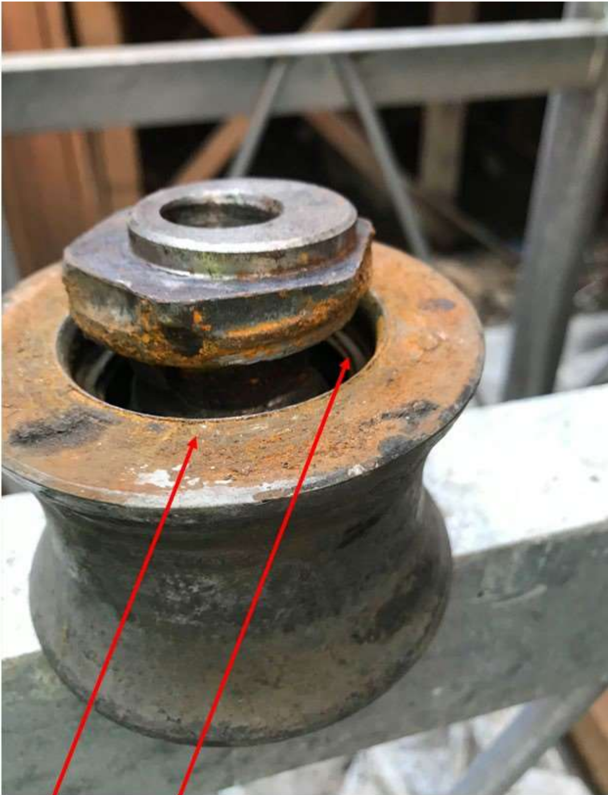
Failed Guide Roller – Bearing Failure
