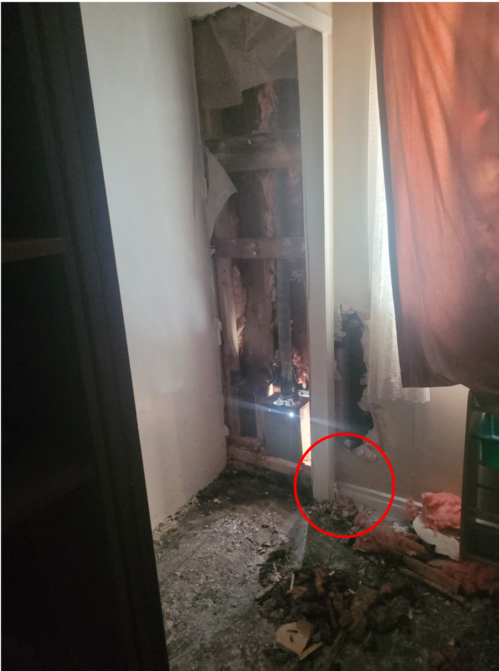
Image 1 - Mast pipe and meter mount prior to removal. Note the electric arcing damage, evidenced by ambient light, where the mast pipe is secured to the meter mount (circled).
