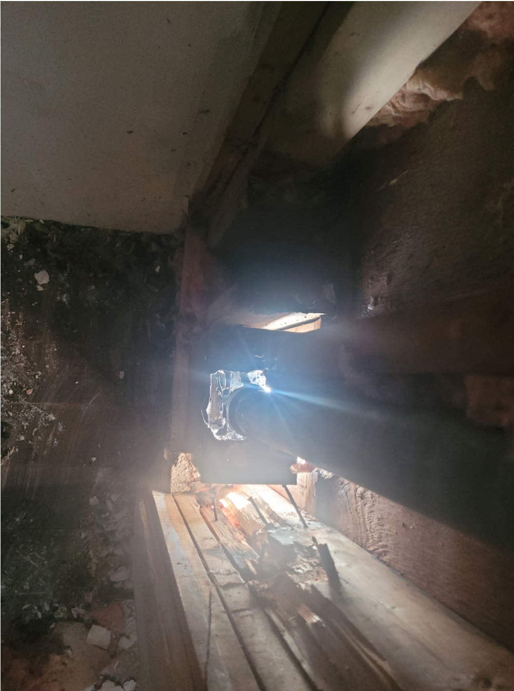
Image 2 - Mast pipe and meter mount prior to removal – top view of arcing damage and charred adjacent combustible material.
