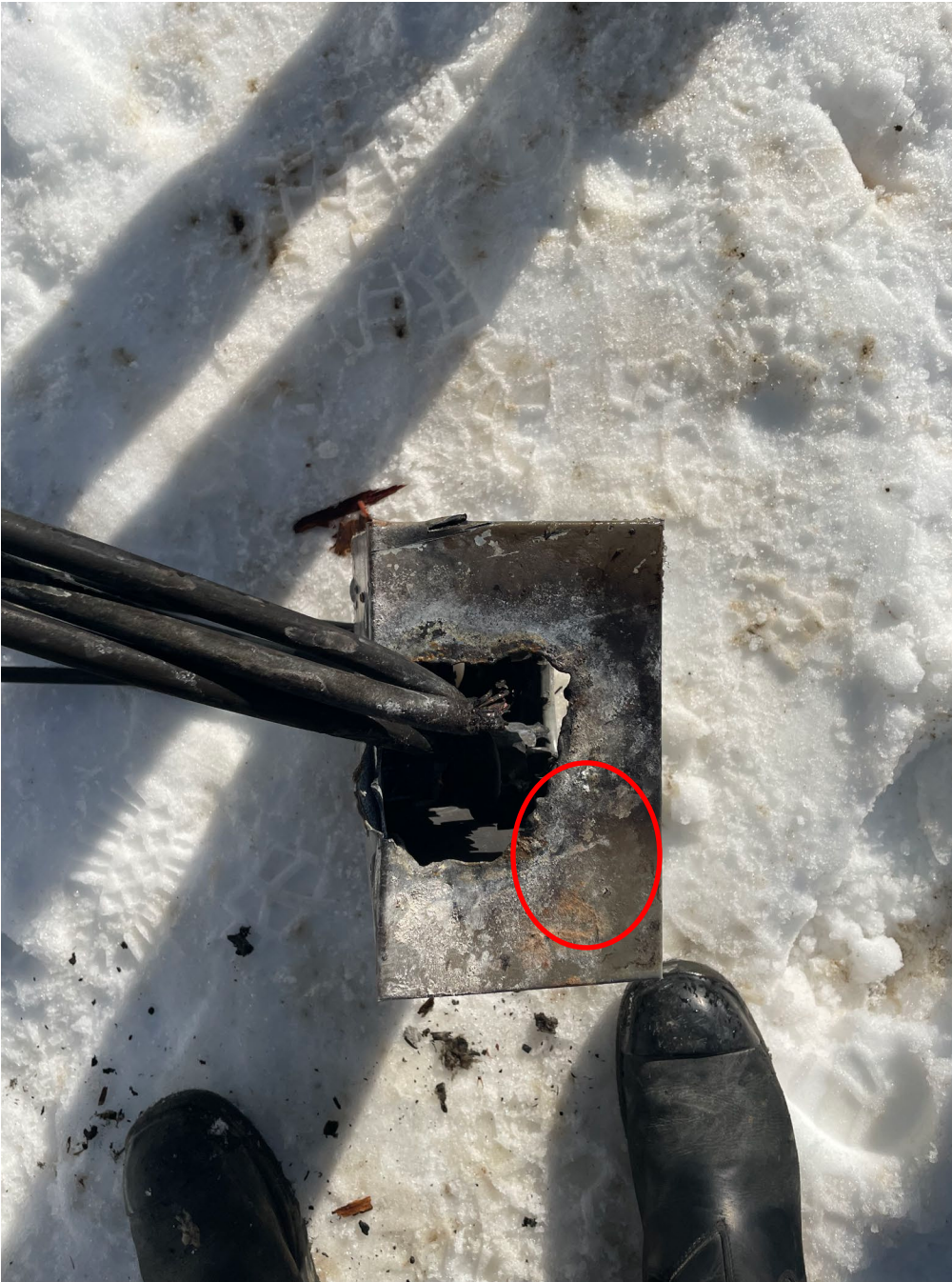
Image 3 - Roof Line: Electric arcing damage to the meter mount enclosure. Circled area indicates the compromised service conductor insulation.
