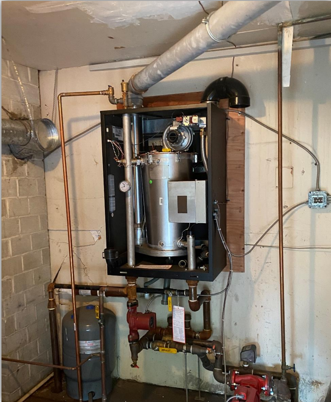
Image 1 – (Maple Ridge incident) Wall hung Boiler in the building mechanical room.
