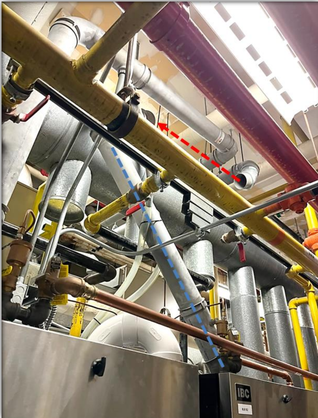
Image 4 – Additional incident ( Appendix A - #4) showing dislodged polypropylene venting from delayed ignitions.
