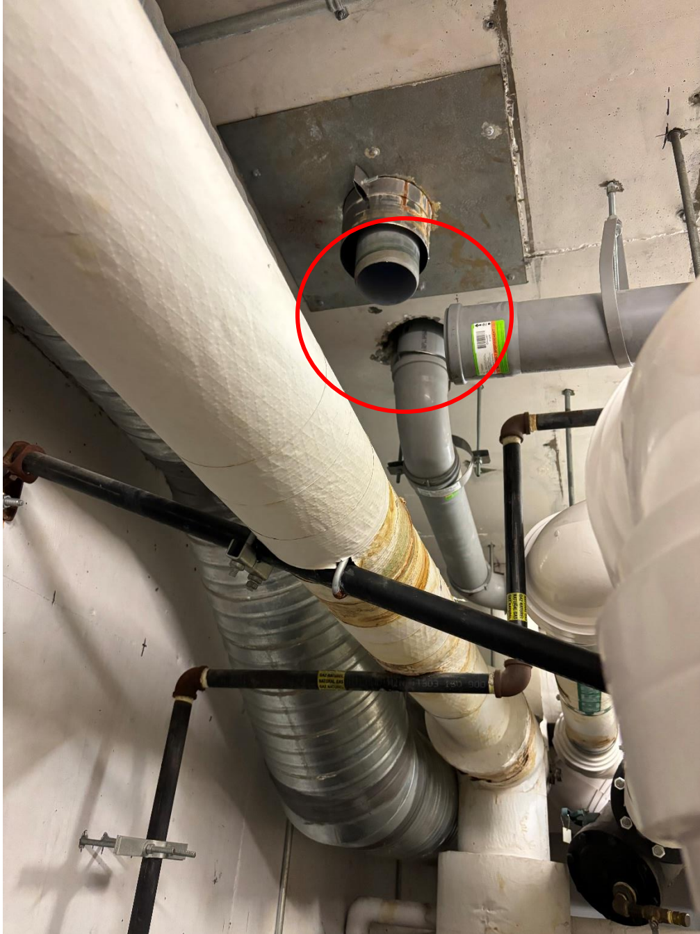
Image 12 - Additional incident ( Appendix A - #11) showing 90-degree polypropylene vent fitting separated from the venting system from delayed ignitions.
