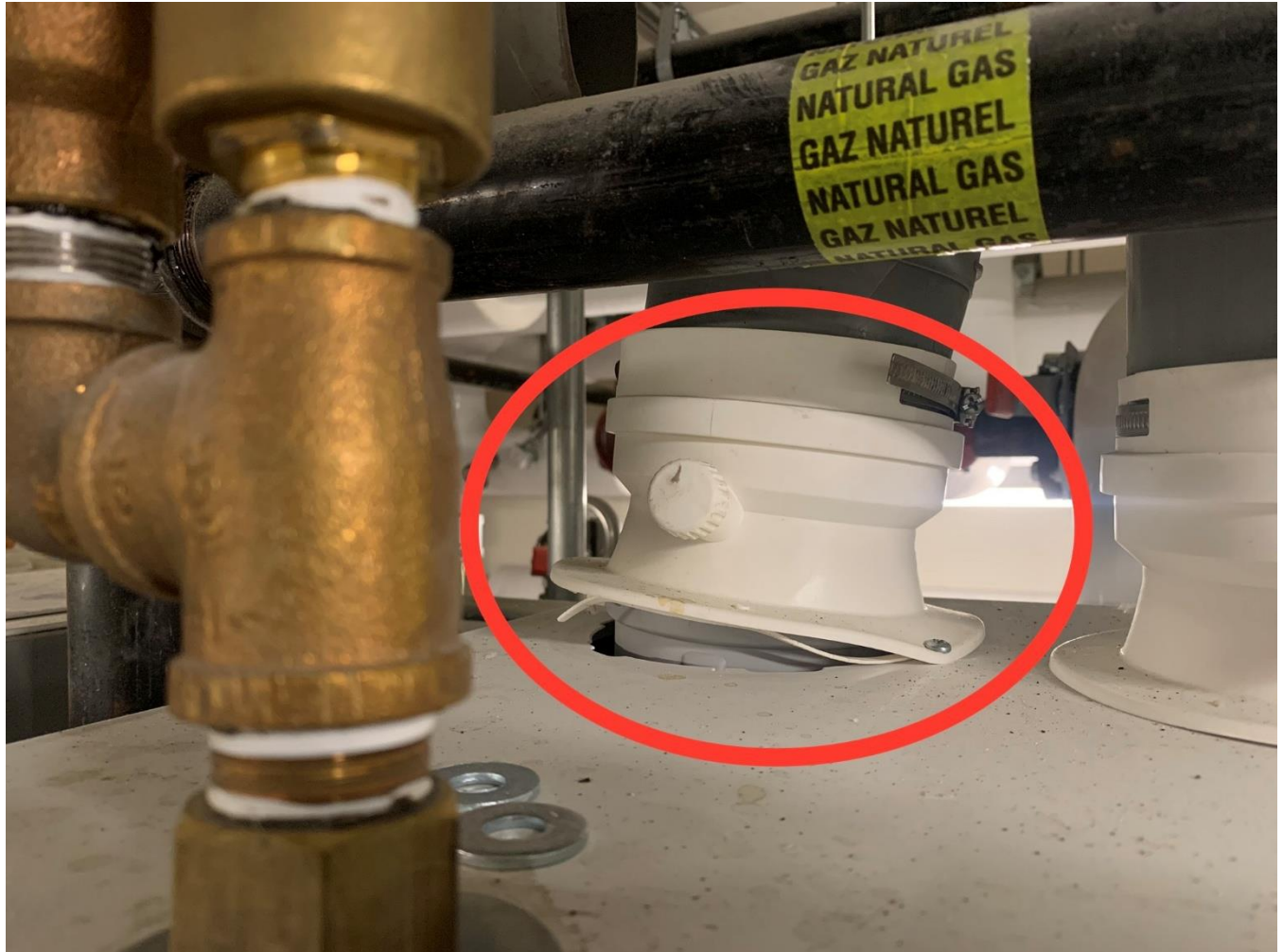
Image 7 - Additional incident ( Appendix A - #7) showing vent output adapter dislodged from the boiler enclosure from delayed ignitions.
