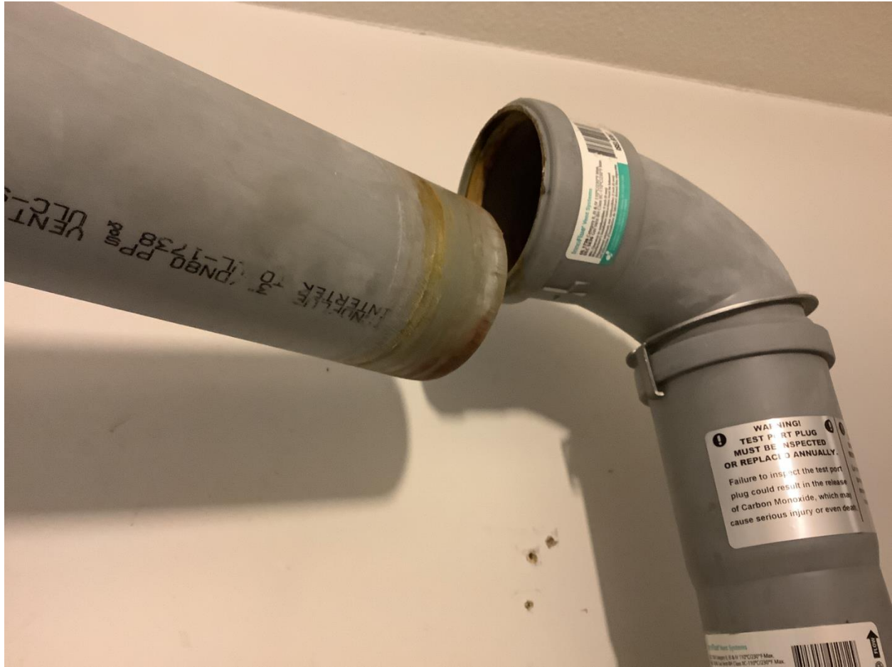
Image 13 - Additional incident ( Appendix A - #10) showing polypropylene venting dislodged from delayed ignitions.
