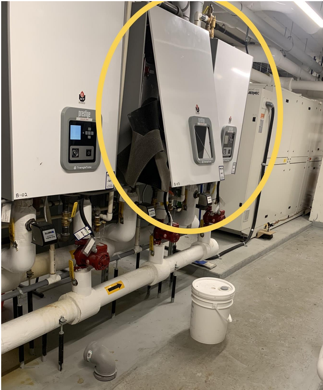
Image 9 - Additional incident ( Appendix A - #7) showing boiler cover blown open from delayed ignitions.
