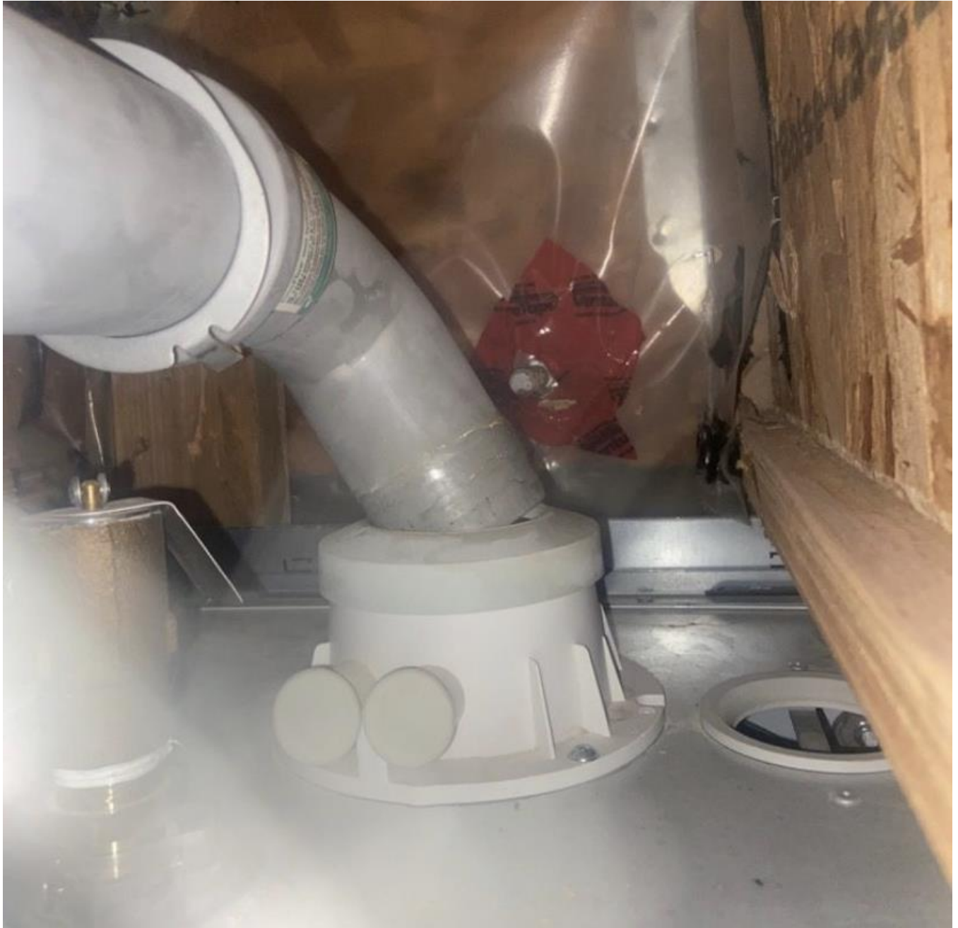
Image 11 - Additional incident ( Appendix A - #9) showing polypropylene venting dislodged from boiler vent connection from delayed ignitions.
