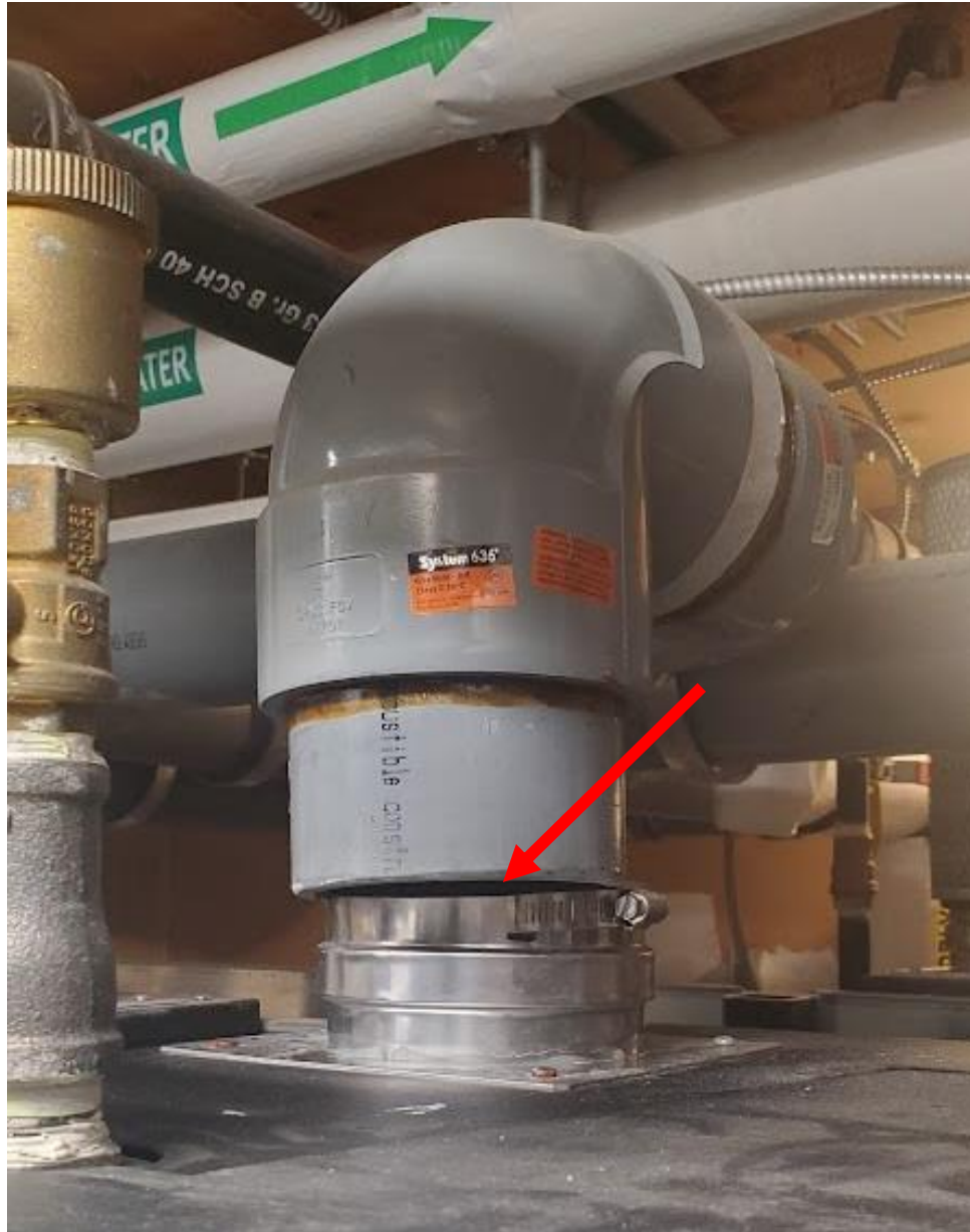
Image 6 - Additional incident ( Appendix A - #5) showing CPVC venting dislodged from boiler vent connection from delayed ignitions.
