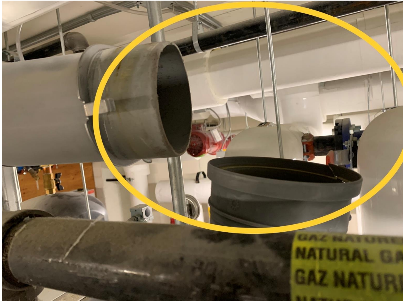
Image 8 - Additional incident ( Appendix A - #7) showing 90-degree polypropylene vent fitting missing from the venting system at the top of the boiler and cracked vent piping from delayed ignitions.
