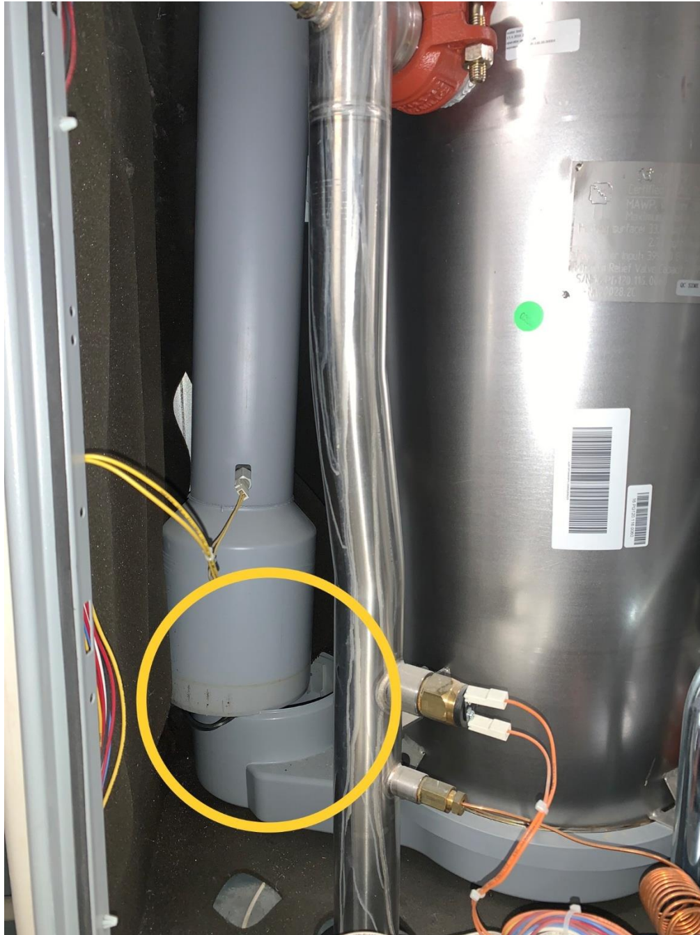
Image 10 - Additional incident ( Appendix A - #7) showing the internal venting output pipe dislodged from the condensate pan from delayed ignitions.
