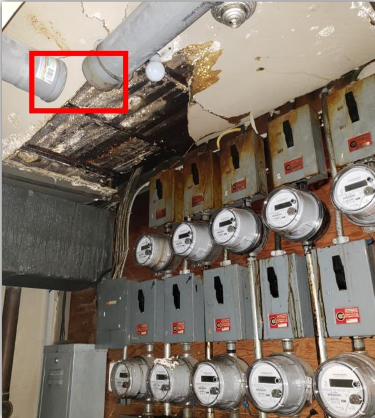
Image 3 – (Maple Ridge incident) Tenant captured image of a missing vent elbow along with the damaged and mouldy drywall above the electrical meters from the sustained operation of the boiler after a delayed ignition damaged the venting.
