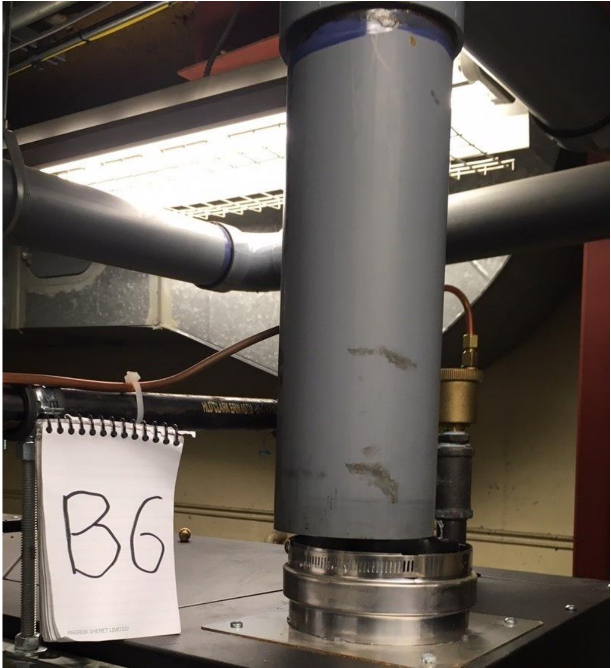
Image 5 - Additional incident ( Appendix A - #1) showing CPVC venting dislodged from boiler vent connection from delayed ignitions.
