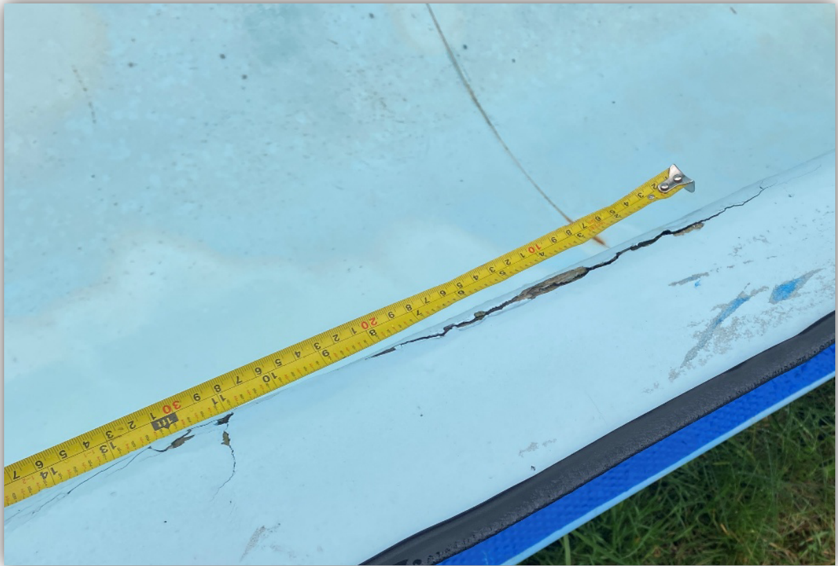
Image 15 - A cracked fiberglass pool edge.
