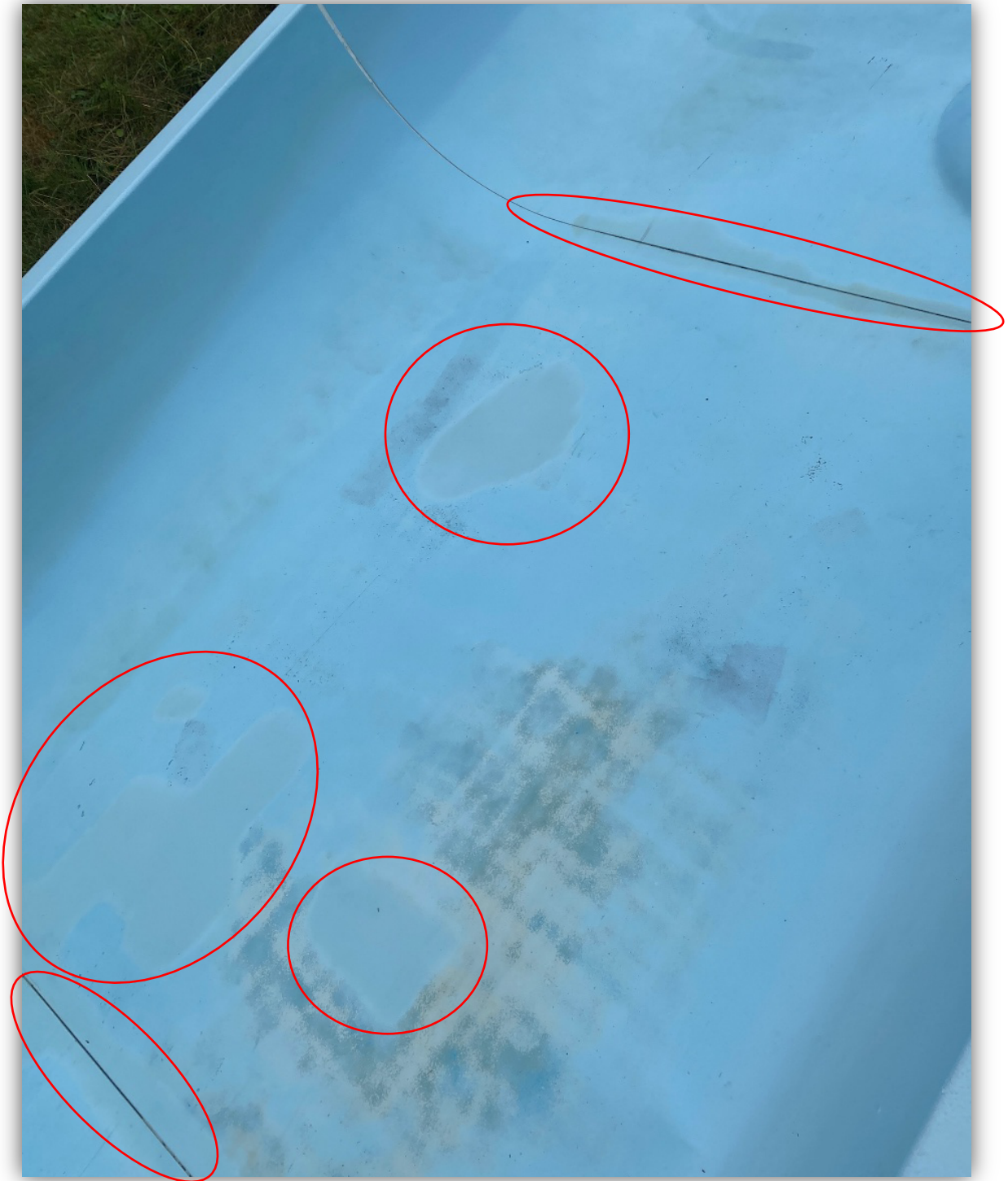
Image 4 – Patched areas of the flume near the failure.
