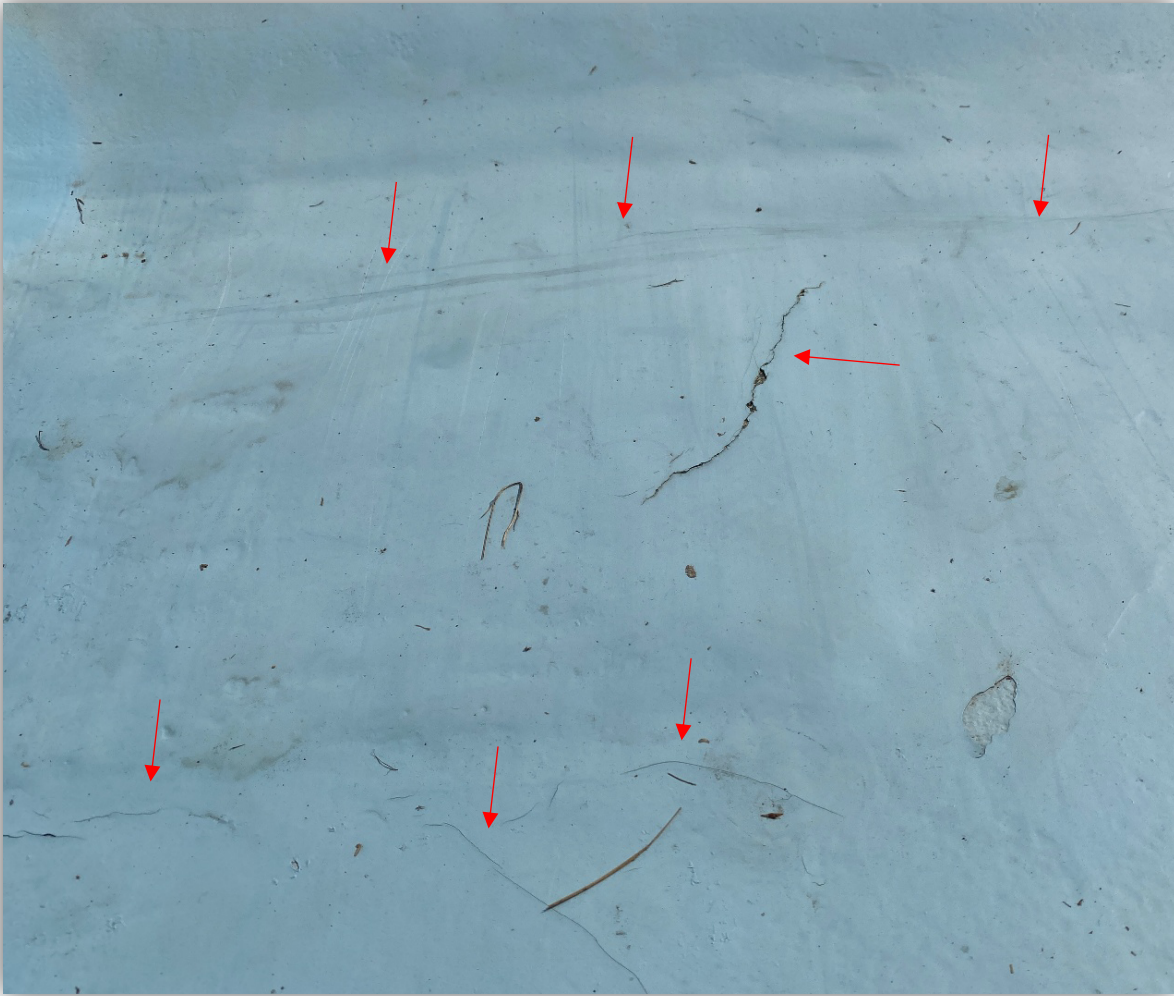
Image 11 – Close-up of the cracked flume section.
