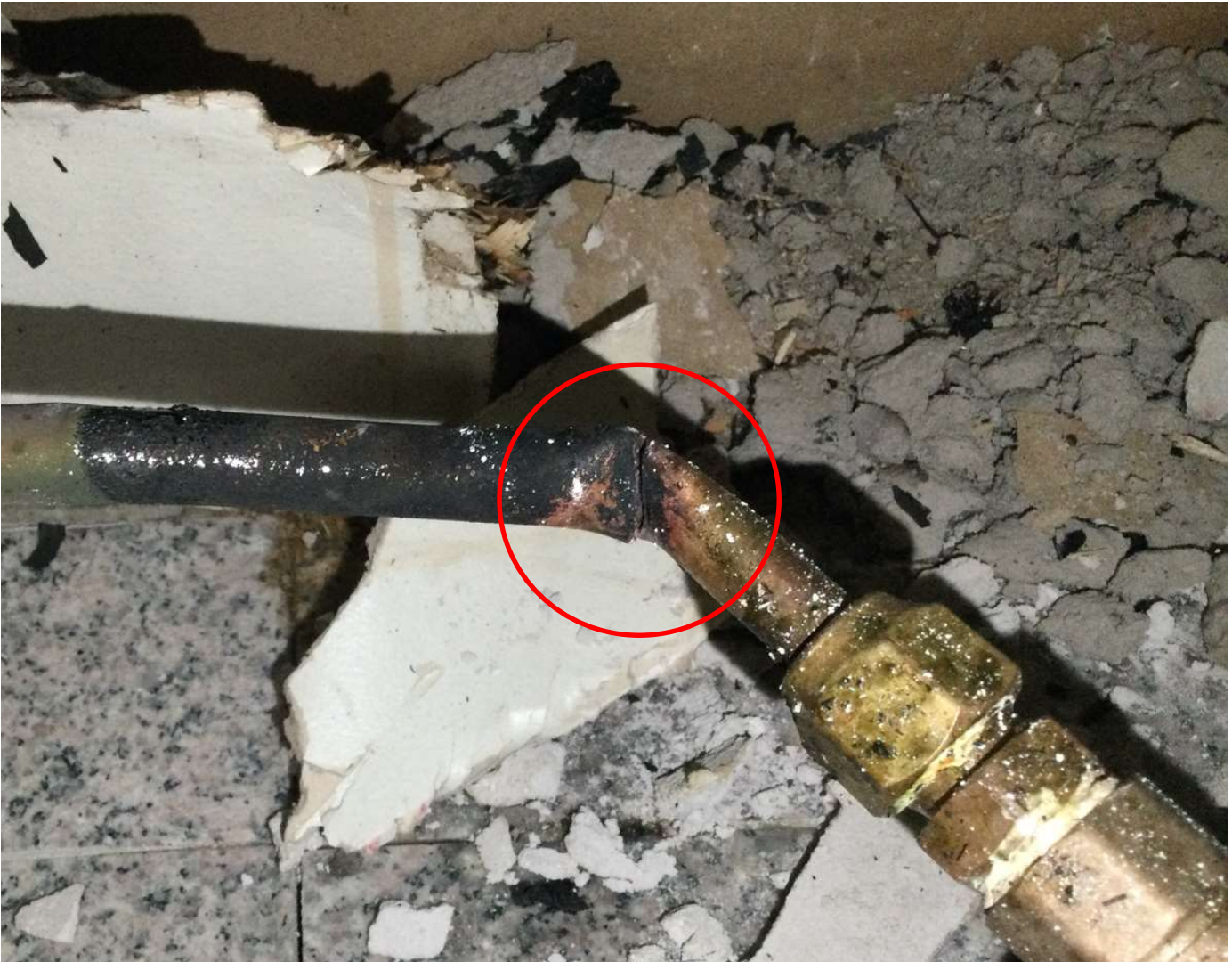
Picture 3- Close examination of the copper tubing shows a break where the tubing was kinked/creased.
