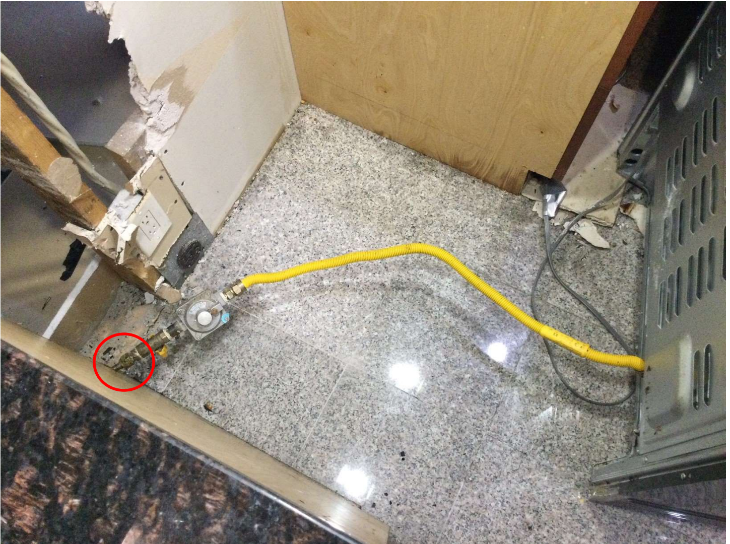
Picture 2- The flexible gas connector can be seen connected to the gas supply. The piping/ regulator was not clamped to the rear wall, this caused the assembly to pull forward straining the copper tubing against the edge of the cabinet. (copper tubing against cabinet circled in red)
