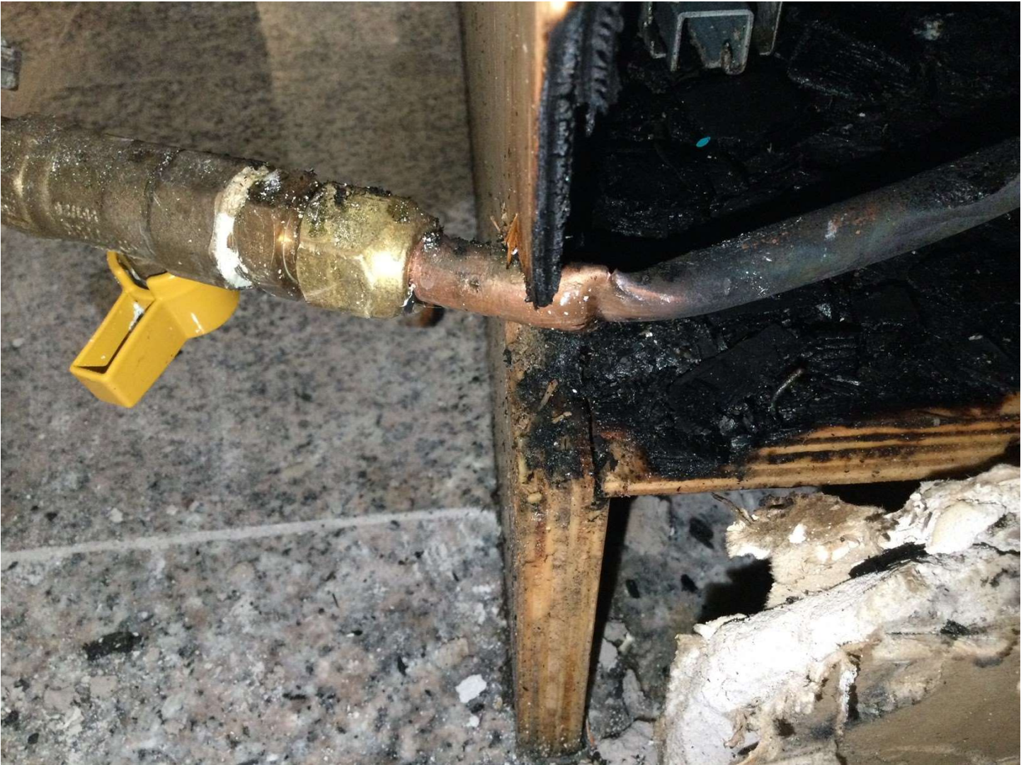
Picture 4- Picture above taken from behind cabinet where the tubing can be seen pushed up tight against the edge of the cabinet.
