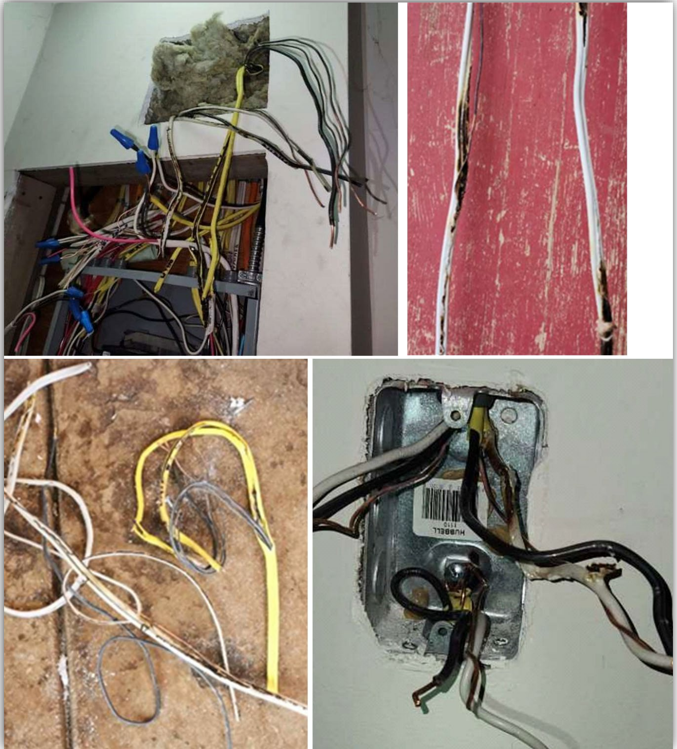
Image 3 - Damaged wiring inside the cabin.
