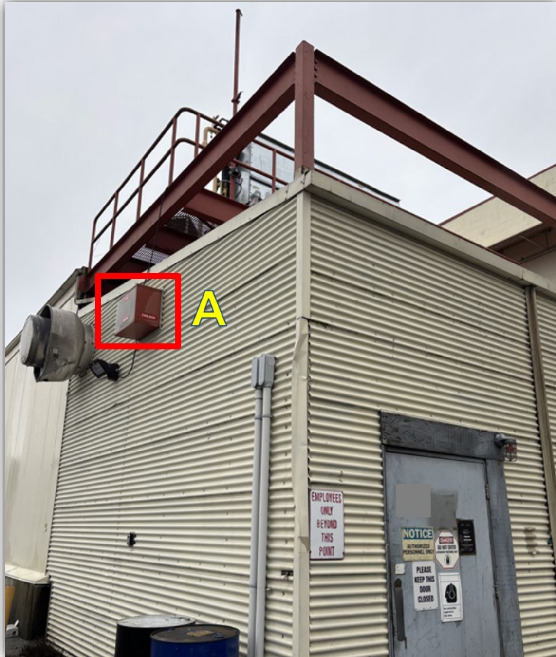
Image 5 – Outside of IQF compressor machine room. [A] The “Fire Box” containing the emergency shutdown for the system accessible only with a ladder and key.
