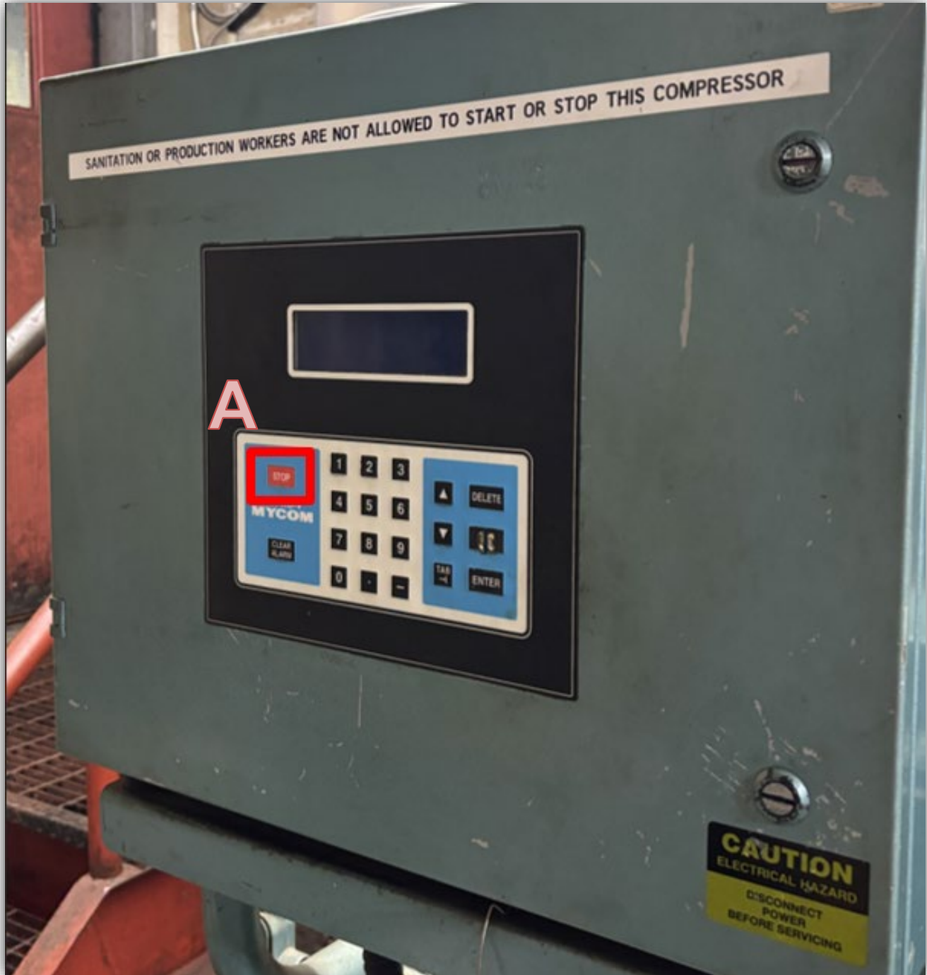
Image 8 – Compressor control panel. [A] The stop button that did not shut down the compressor when pushed.
