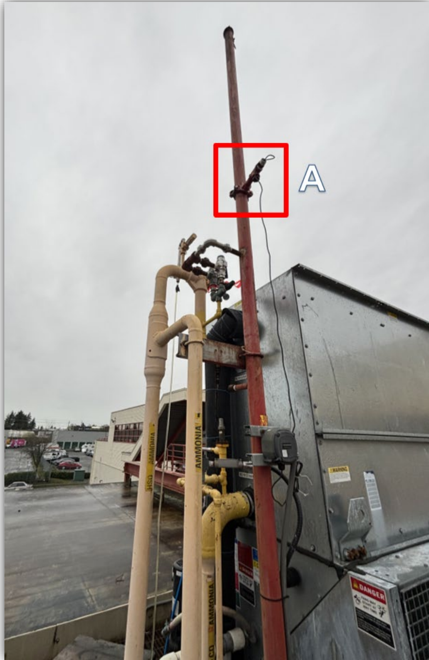
Image 4 – Red relief stack above the compressor machine room. [A] The ammonia detection sensor that alerted the facility of the release.
