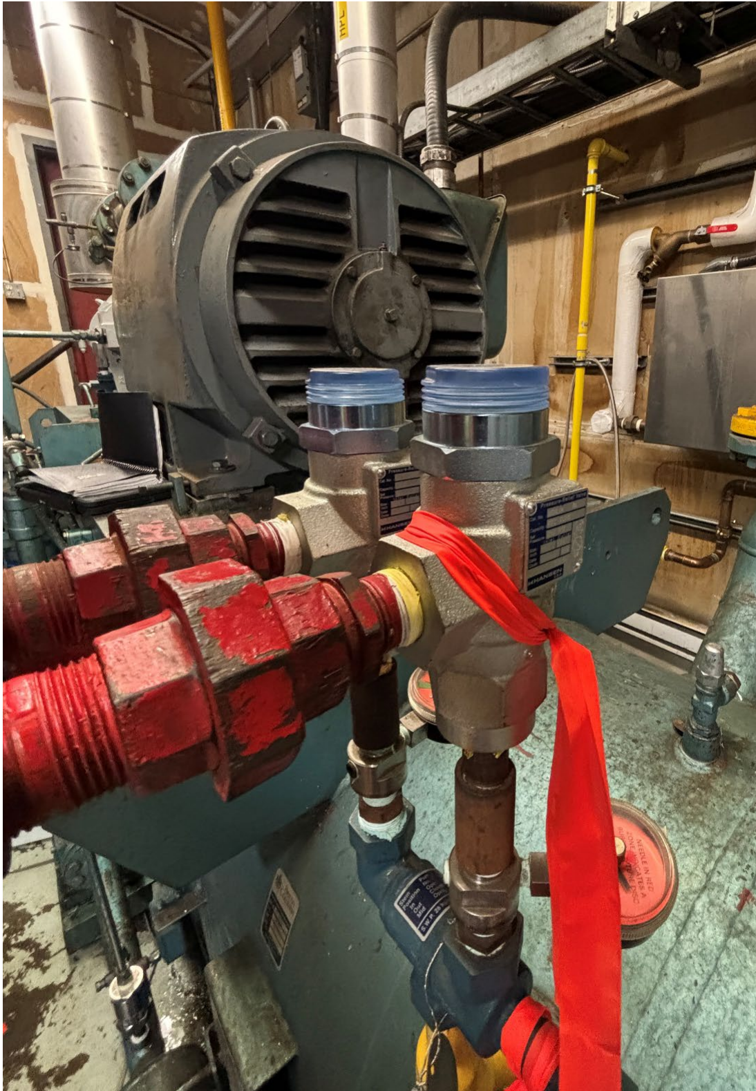
Image 7 – 250 psi pressure relief valves. Red flagging around the valve that opened and released ammonia.
