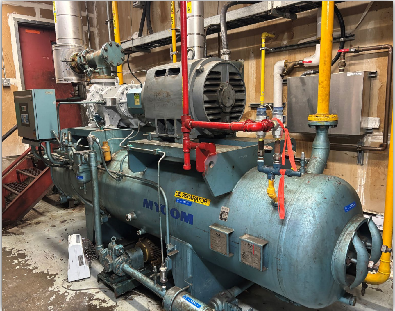
Image 6 – IQF ammonia compressor.
