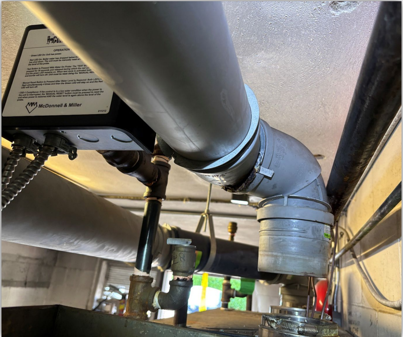
Image 7 – Disconnected vent pipe wedged against external low-water cutoff valve holding it in place.
