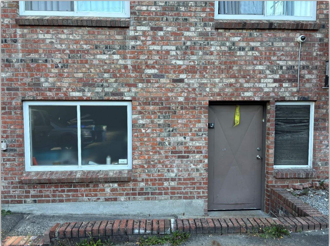
Image 2 – Mechanical room door with passive air intake opening, screen, and louvers on the right side.
