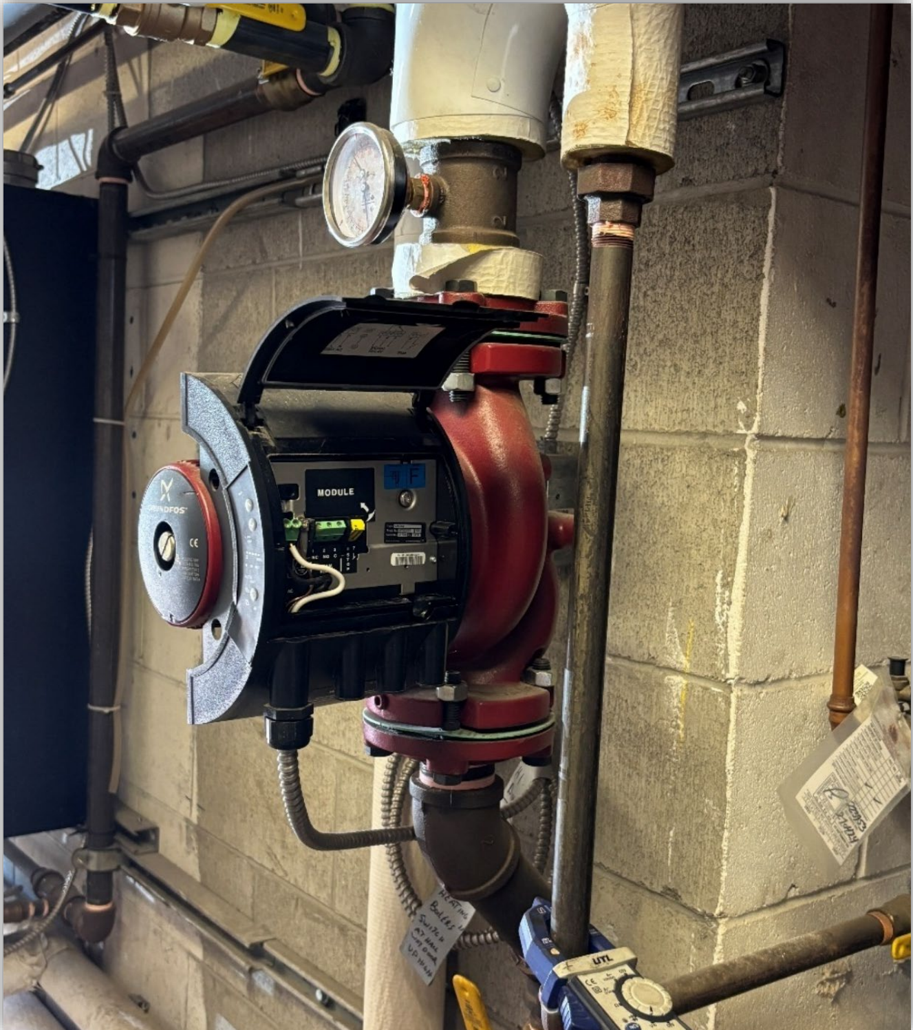
Image 13 – Main circulating pump for building's hydronic heating system.
