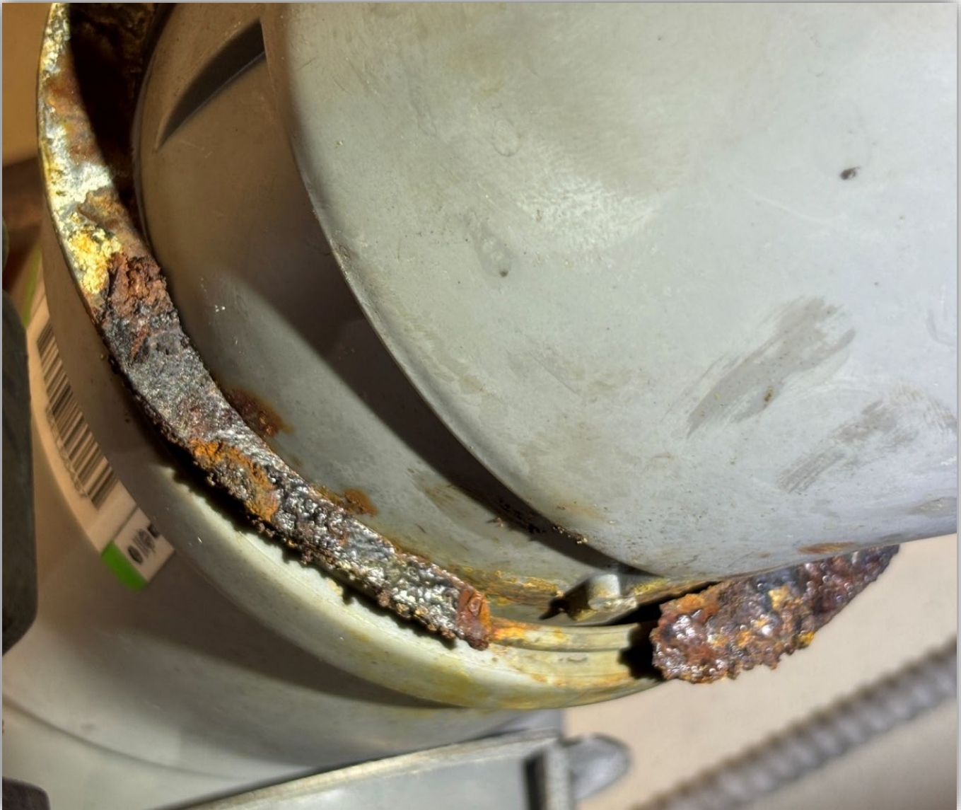
Image 8 – Close-up of corroded retaining ring on Boiler #2 vent elbow.
