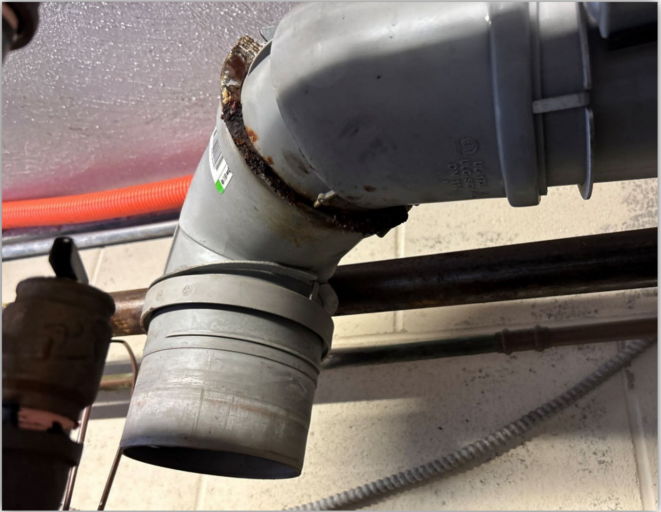
Image 5 – Close-up of disconnected vent and corroded retaining ring.
