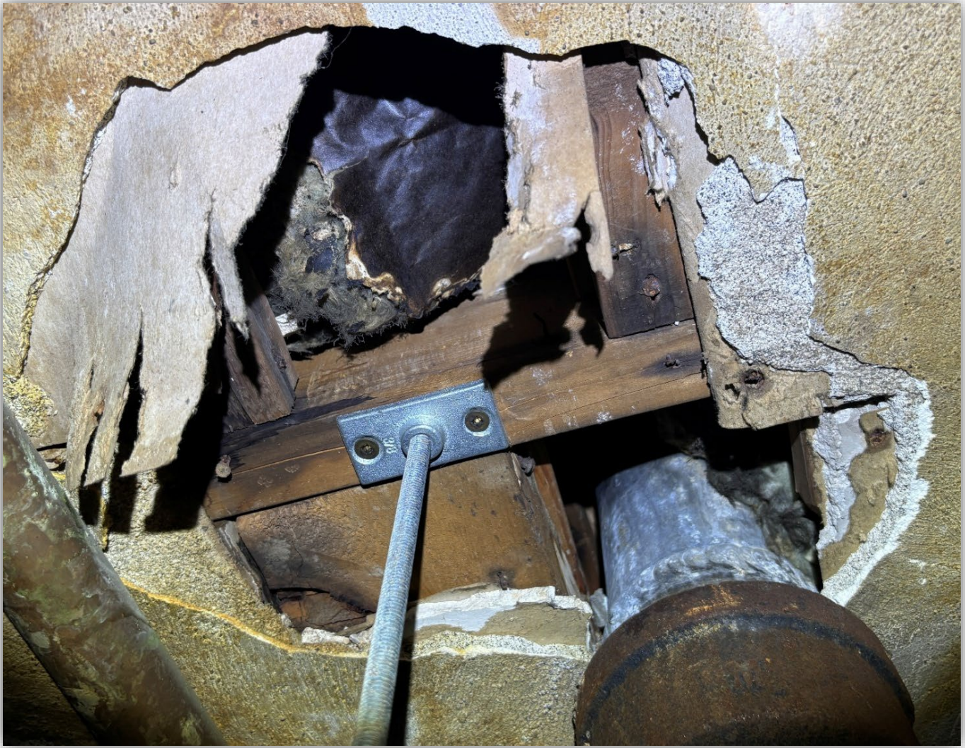
Image 12 – Hole in mechanical room ceiling providing a migration path for CO into the building with vent support bracket installed on exposed floor joist.
