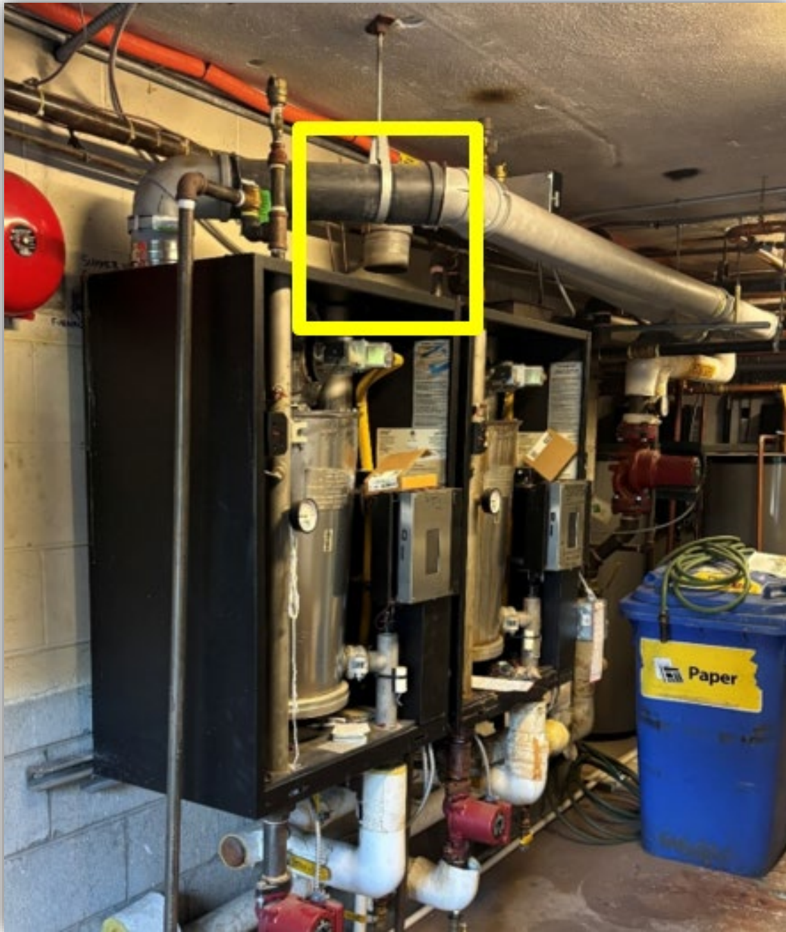
Image 3 – Two heating boilers in the mechanical room, with the disconnected vent on Boiler #2 shown at right.
