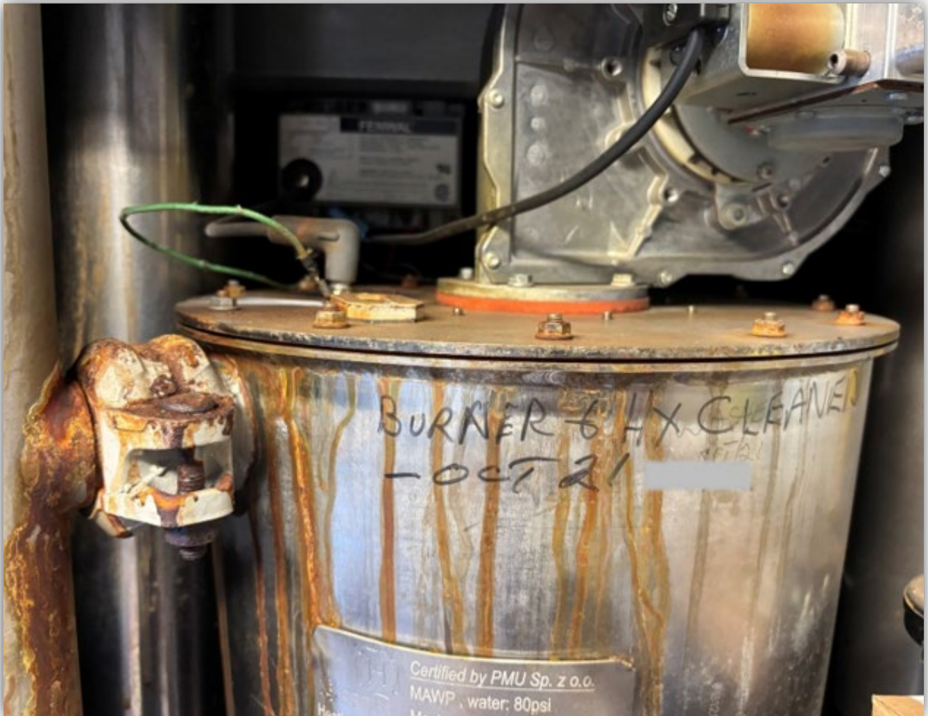
Image 10 – Staining and corrosion on combustion chamber from leaking condensate from flue vent on Boiler #2.
