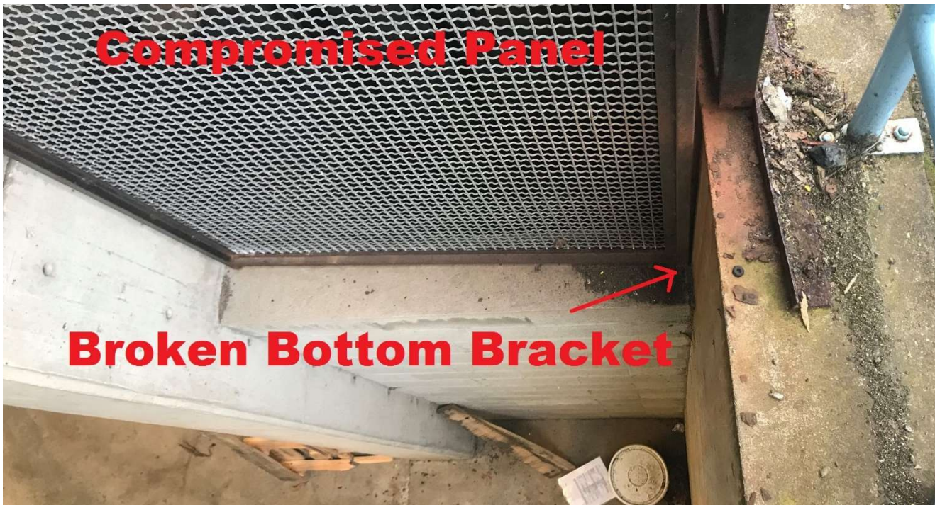
Photo 4 – Broken bottom bracket of compromised enclosure panel
