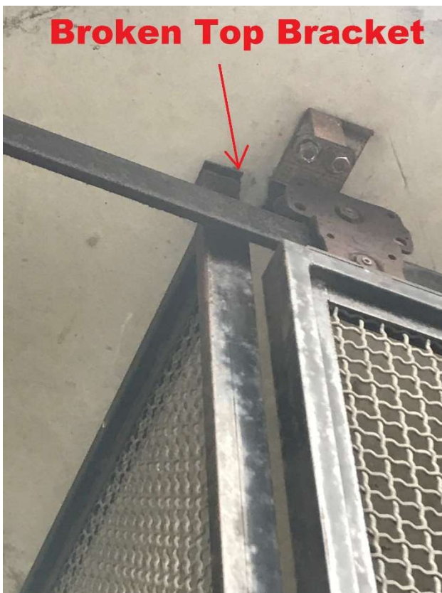
Photo 3 – Broken top bracket of compromised enclosure panel
