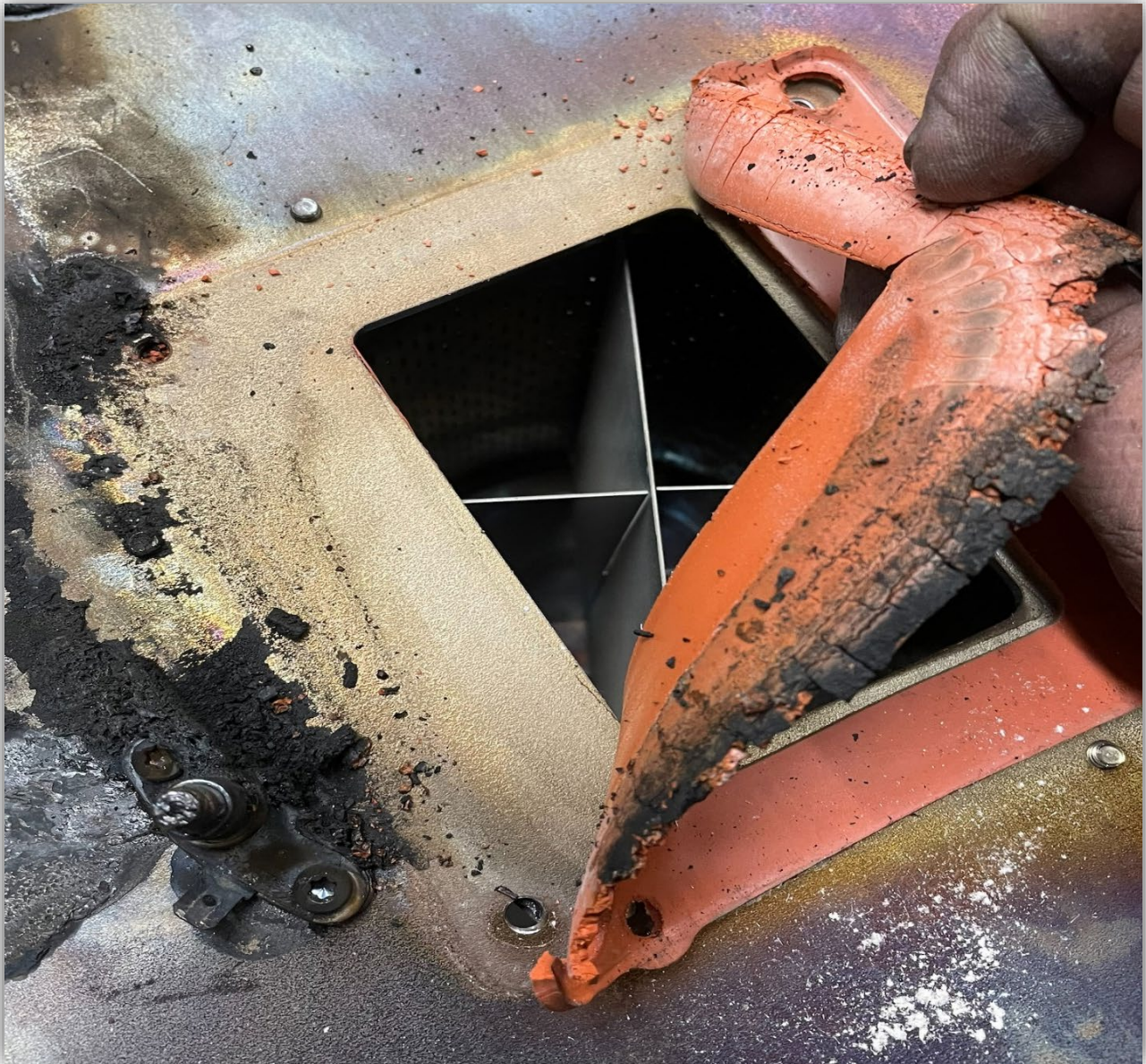
Image 4 - Fan motor gasket (orange) where combustion flame contacted the heat exchanger lid. Hot combustion gases escaped through the heat exchanger lid gasket melting the fan motor and exposing heat and smoke to the gas assembly.
