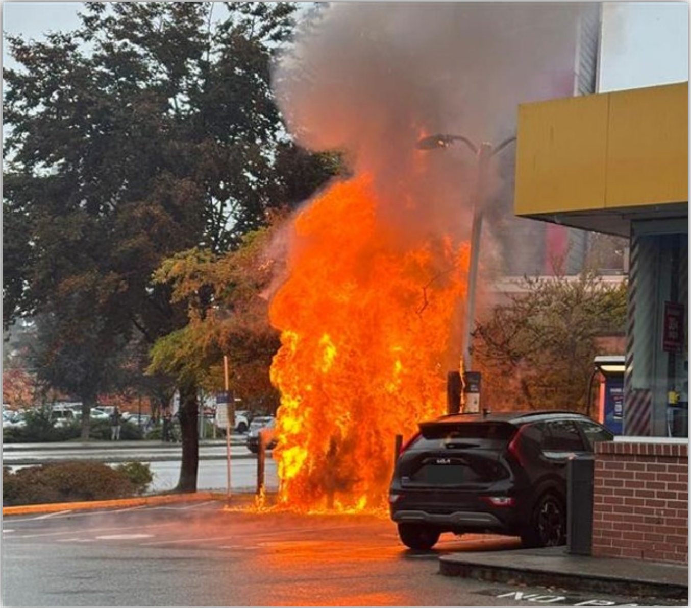
Image 1 – EV charger on fire at retail charging location.
