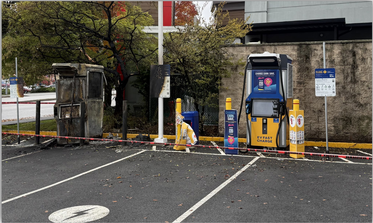
Image 2 – Damaged charger and surrounding area after incident.
