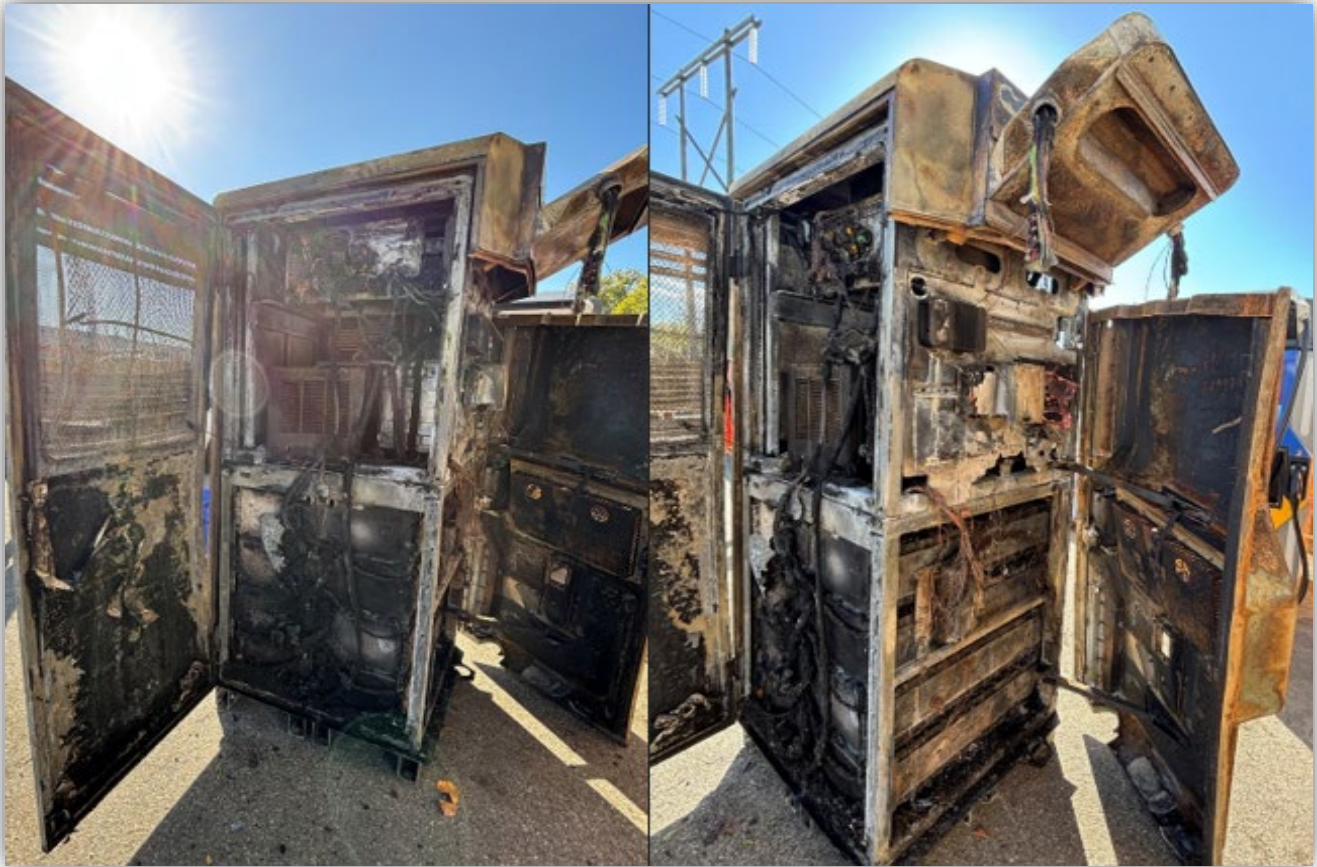
Image 3 – Damaged charger after removal from site.
