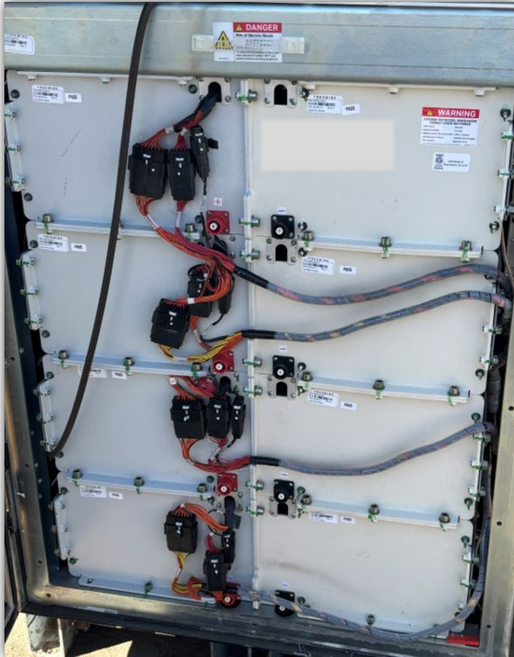
Image 4 – Example of a battery cube assembly inside a Freewire Boost charger showing eight individual module “stacks” bolted together to form one 800V DC lithium-ion battery (Connecting battery jumpers removed).
