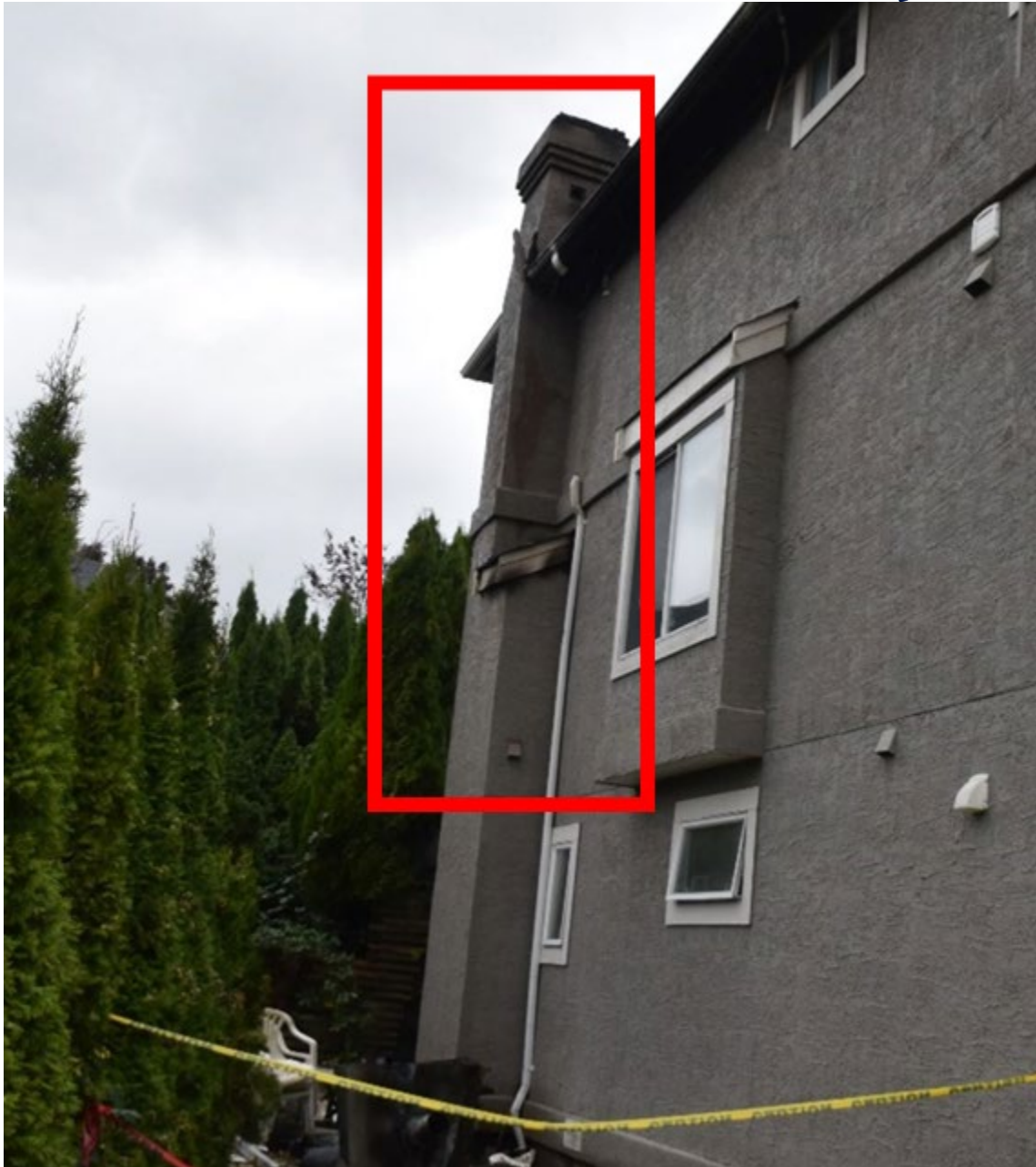
Photo 2 – RED box showing gas fireplace venting chase after the incident.
