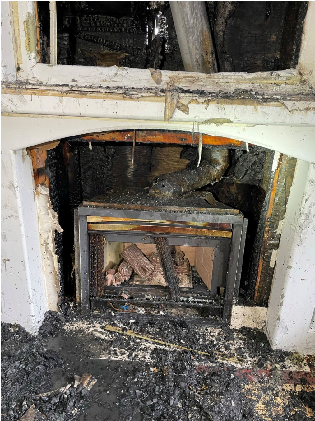
Photo 4 - Gas fireplace showing fire damage and collapsed venting.
