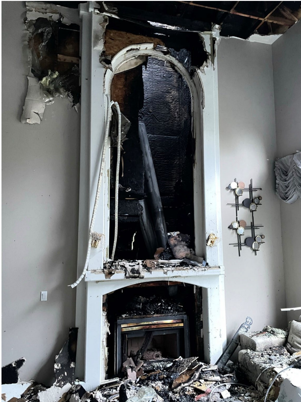
Photo 3 – Gas fireplace and damaged venting and vent chase.
