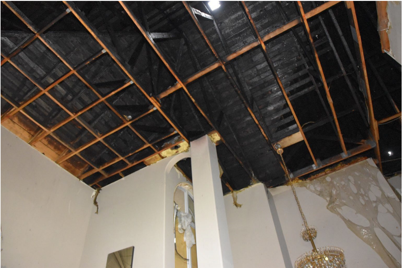
Photo 9 – Ceiling space above the fireplace showing the result of the explosion forcing the drywall and insulation down and subsequent fire damage.
