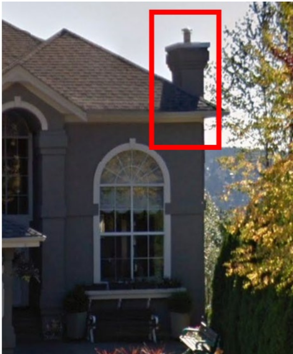
Photo 1 – Street View from Google Maps with RED box showing the fireplace venting before the incident.
