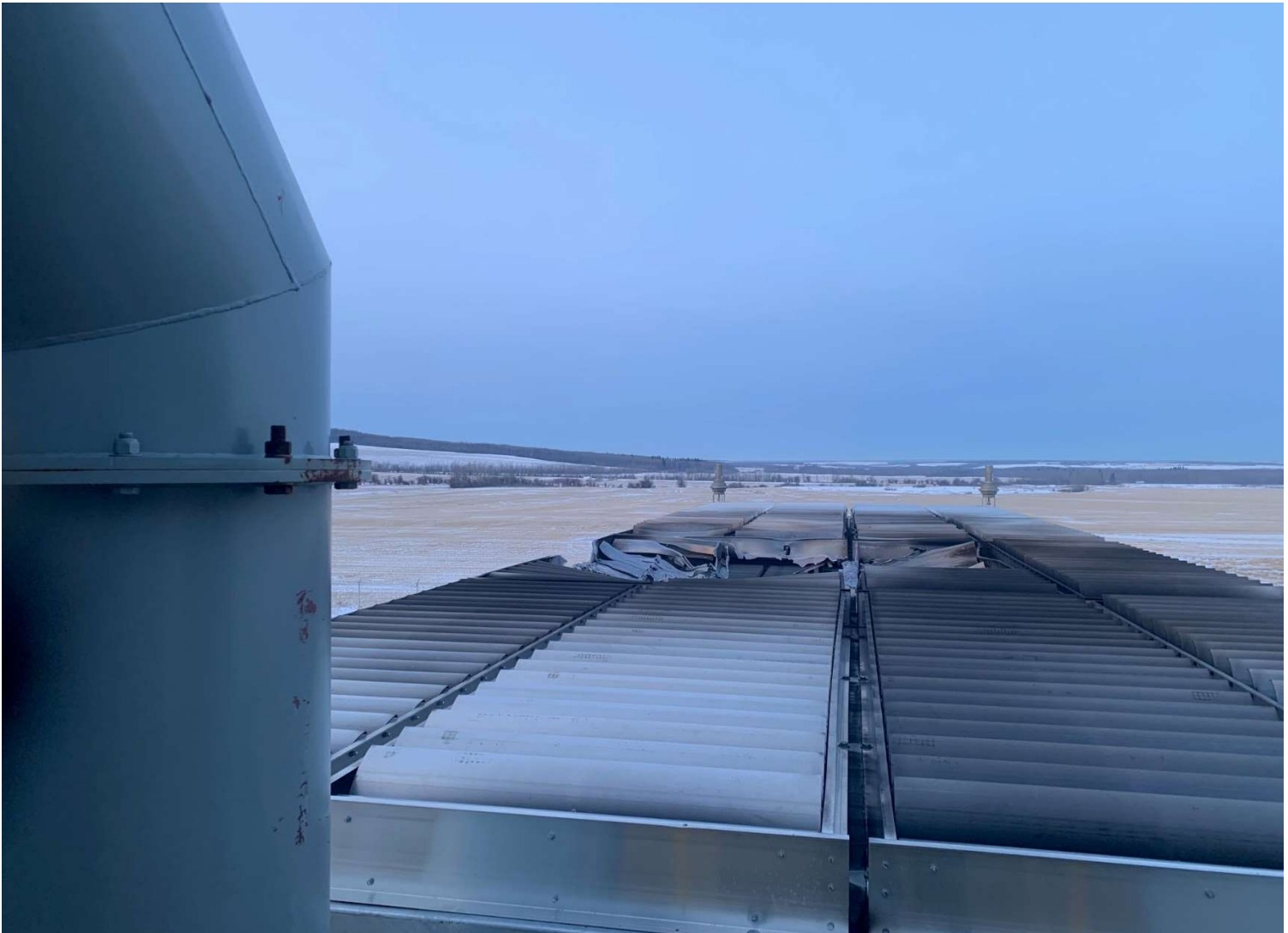
Top of Cooler View
