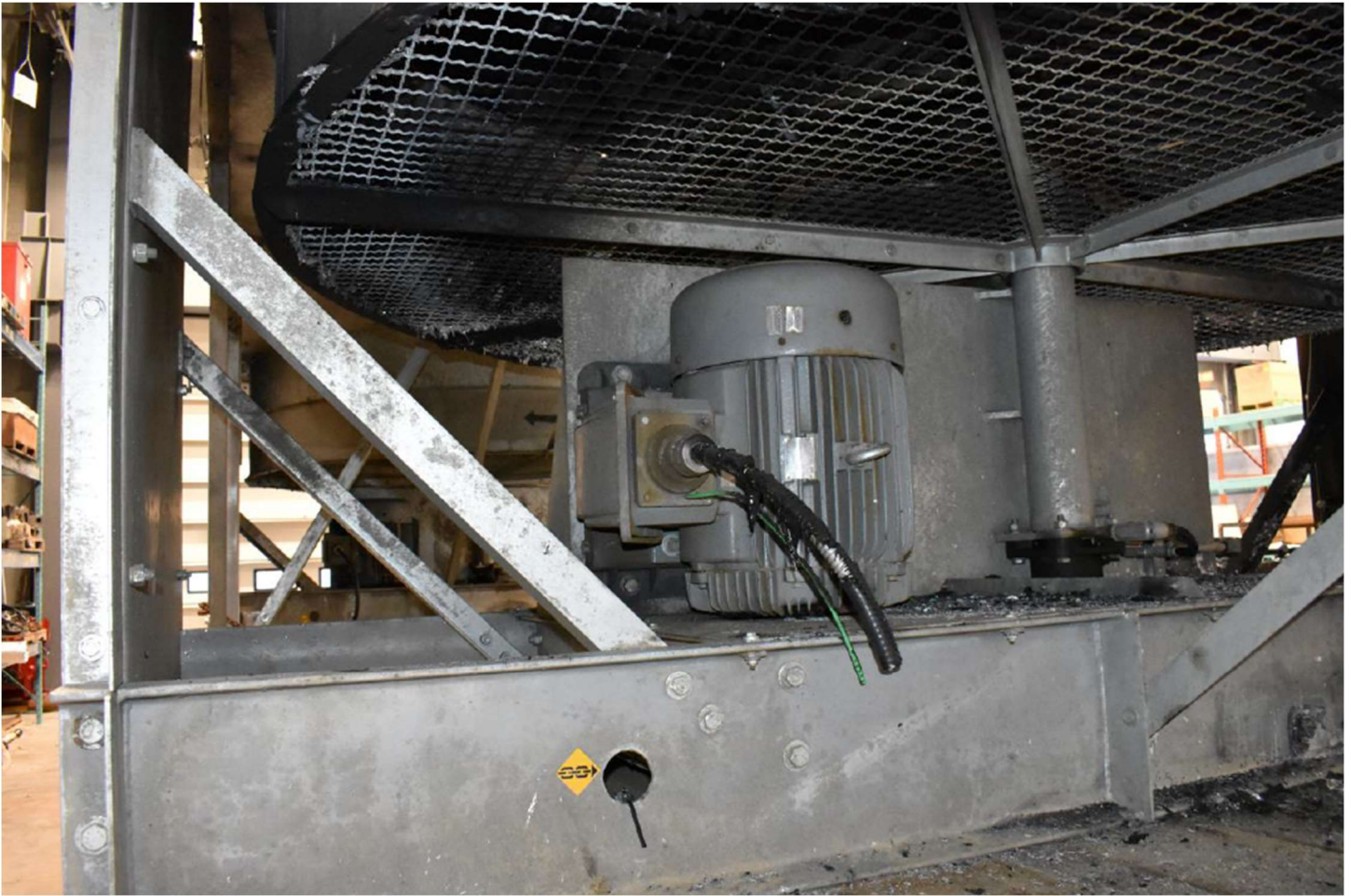
Electric Fan Motor below tubes- wires cut for removal of Cooler
