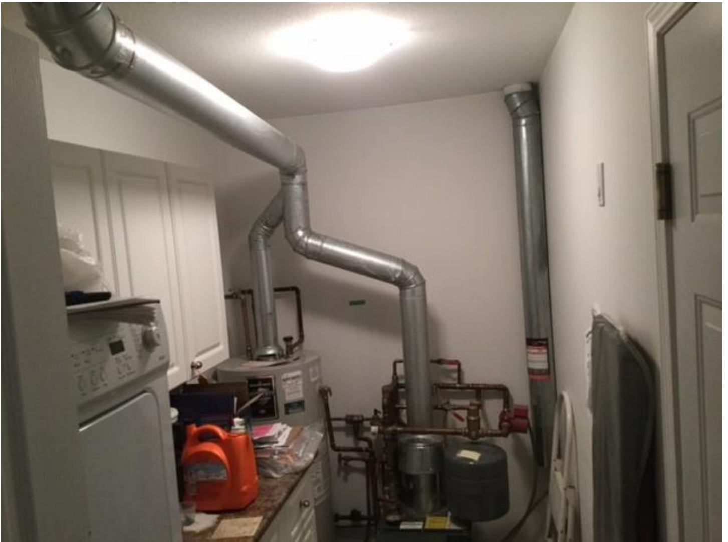
Boiler room and correct venting arrangement.
