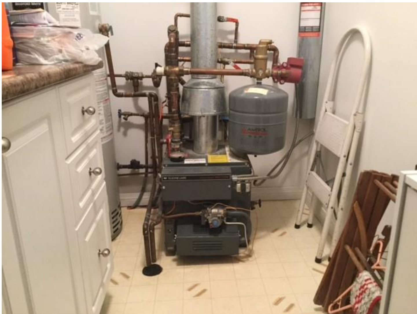
Boiler room/Laundry room in townhouse unit.
