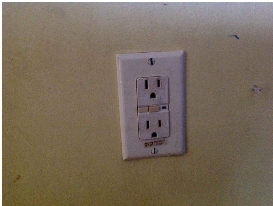
Photo 2: failed receptacle as installed – no evidence of damage when viewed.
