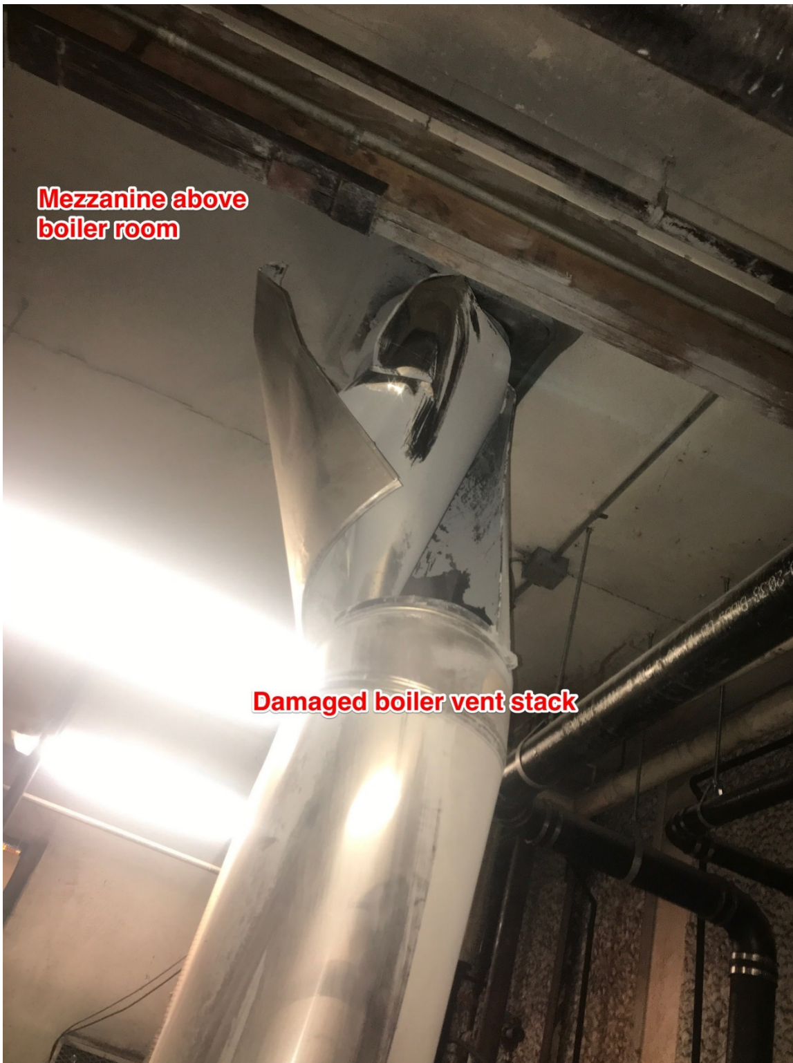
Image 4 - Boiler vent stack above boiler
