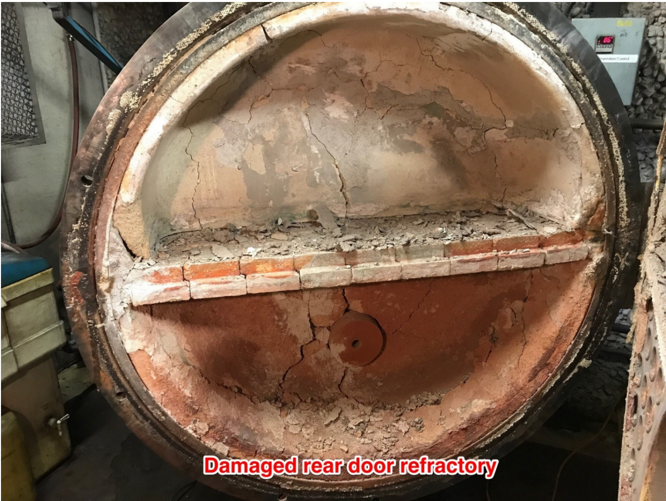
Image 8 - Cracked and broken rear door refractory insulation
