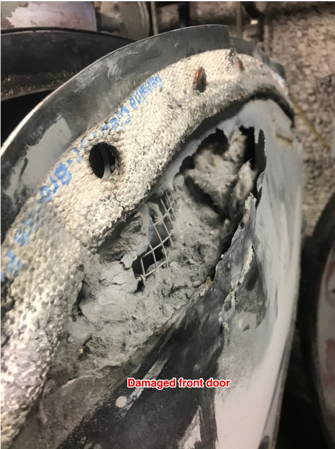
Image 7 - Damage to boiler front door
