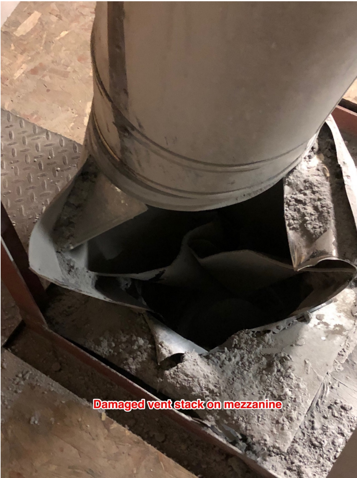
Image 5 - Boiler vent stack at mezzanine above boiler room
