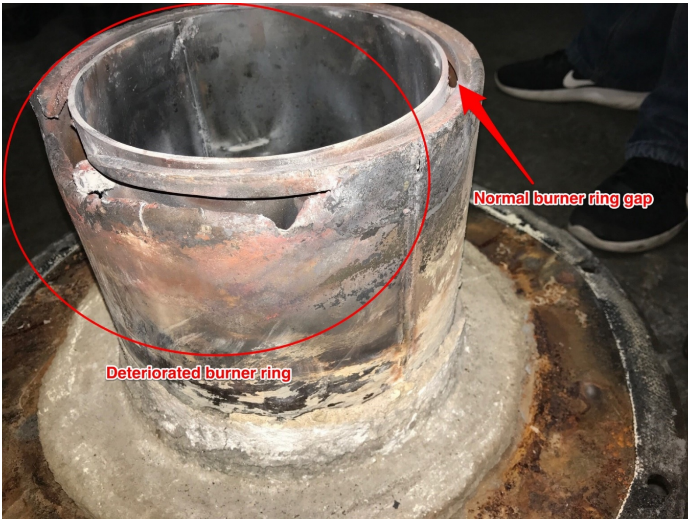
Image 11 - Burner housing with deteriorated ring and large gas port opening
