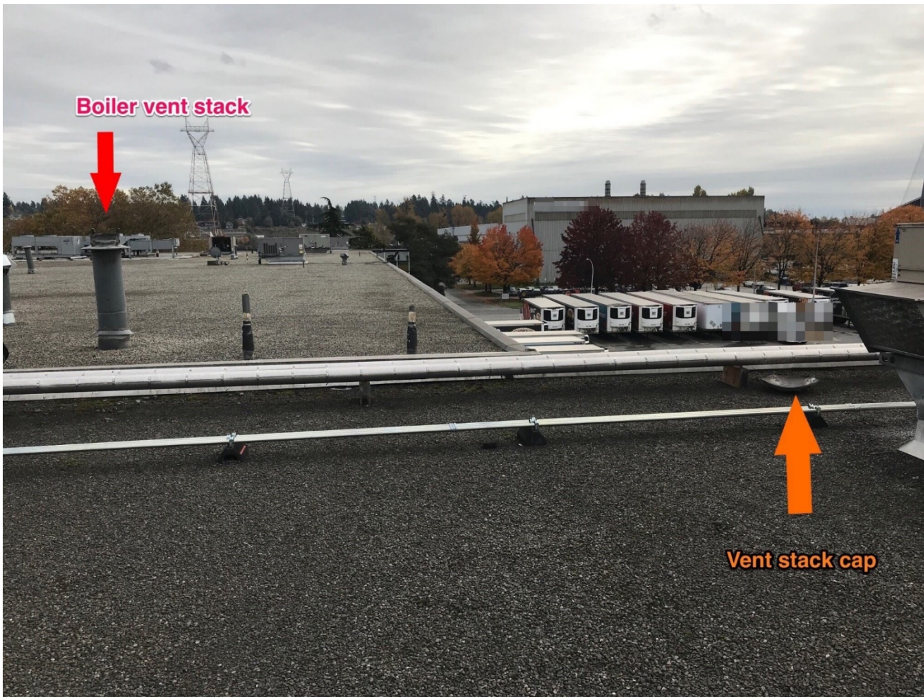
Image 6 - Location of vent cap after it was blown off the boiler vent stack by the explosion
