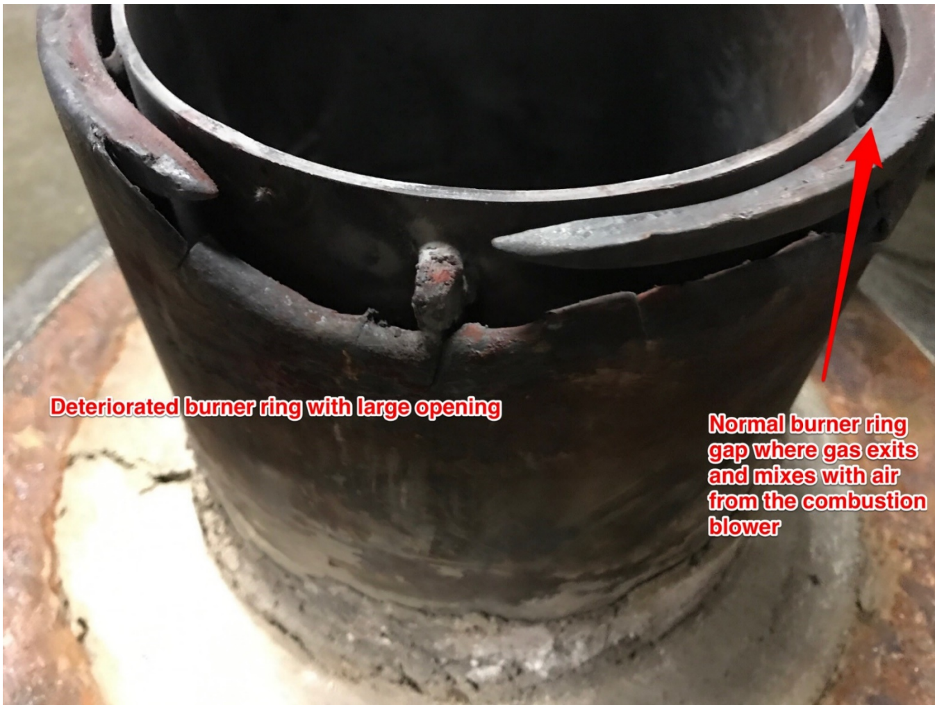
Image 10 - Burner housing with deteriorated ring and large gas port opening. The air diffuser gets positioned in the middle circular area of the burner housing.
