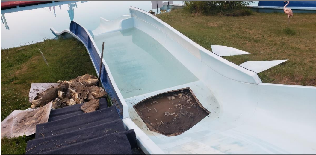
Figure 2 Area of cut out fibreglass showing deteriorated foam under cracked panel.
