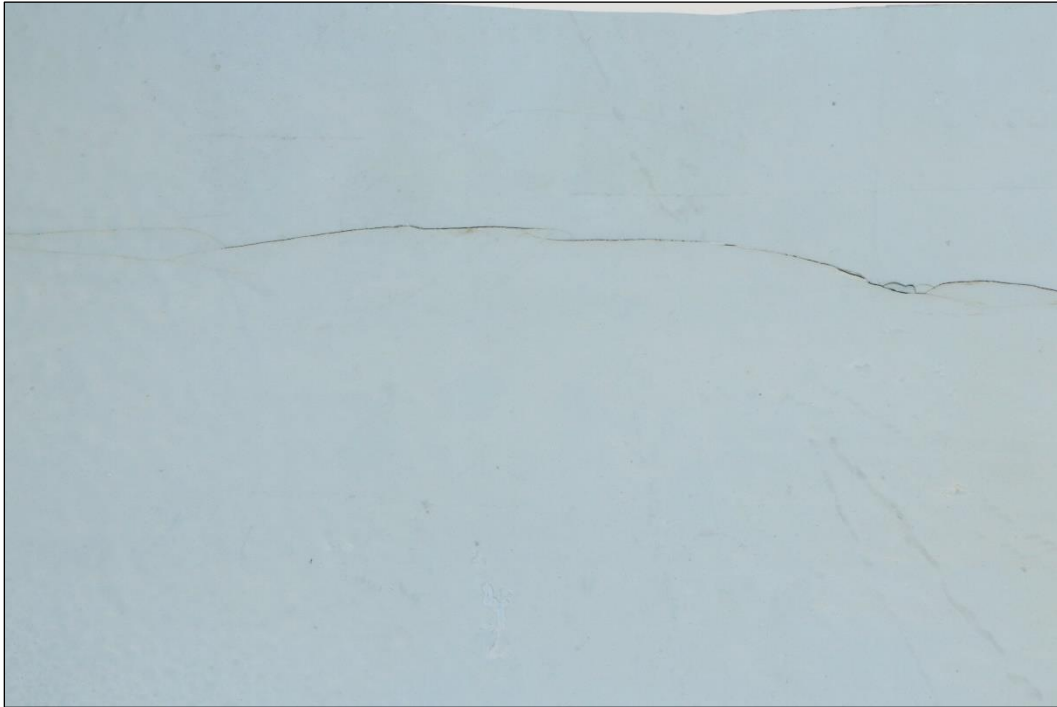
Figure 16 Closer view of crack on sample F.
