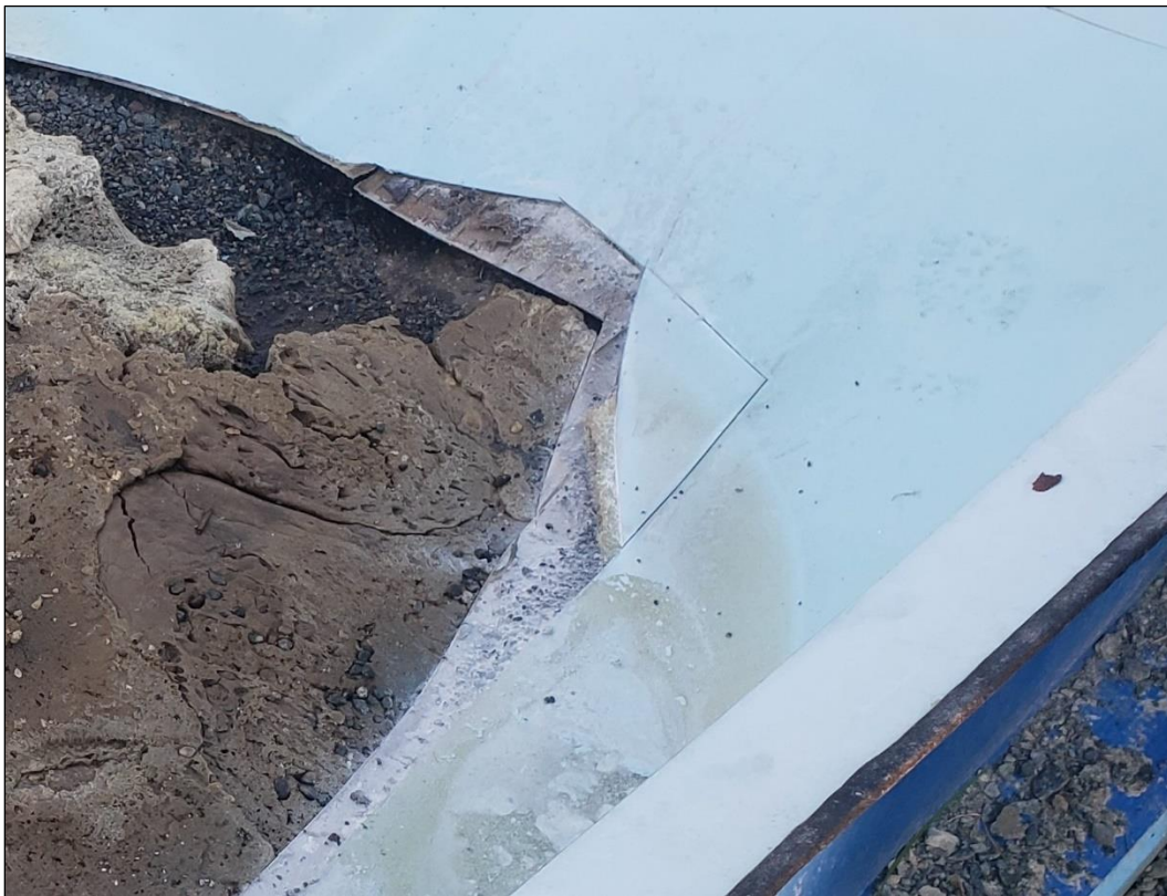
Figure 3 Cut is slide near fracture showing slide construction with wood core and an inner and outer layer of fibreglass. Underlying dark material is injected foam.
