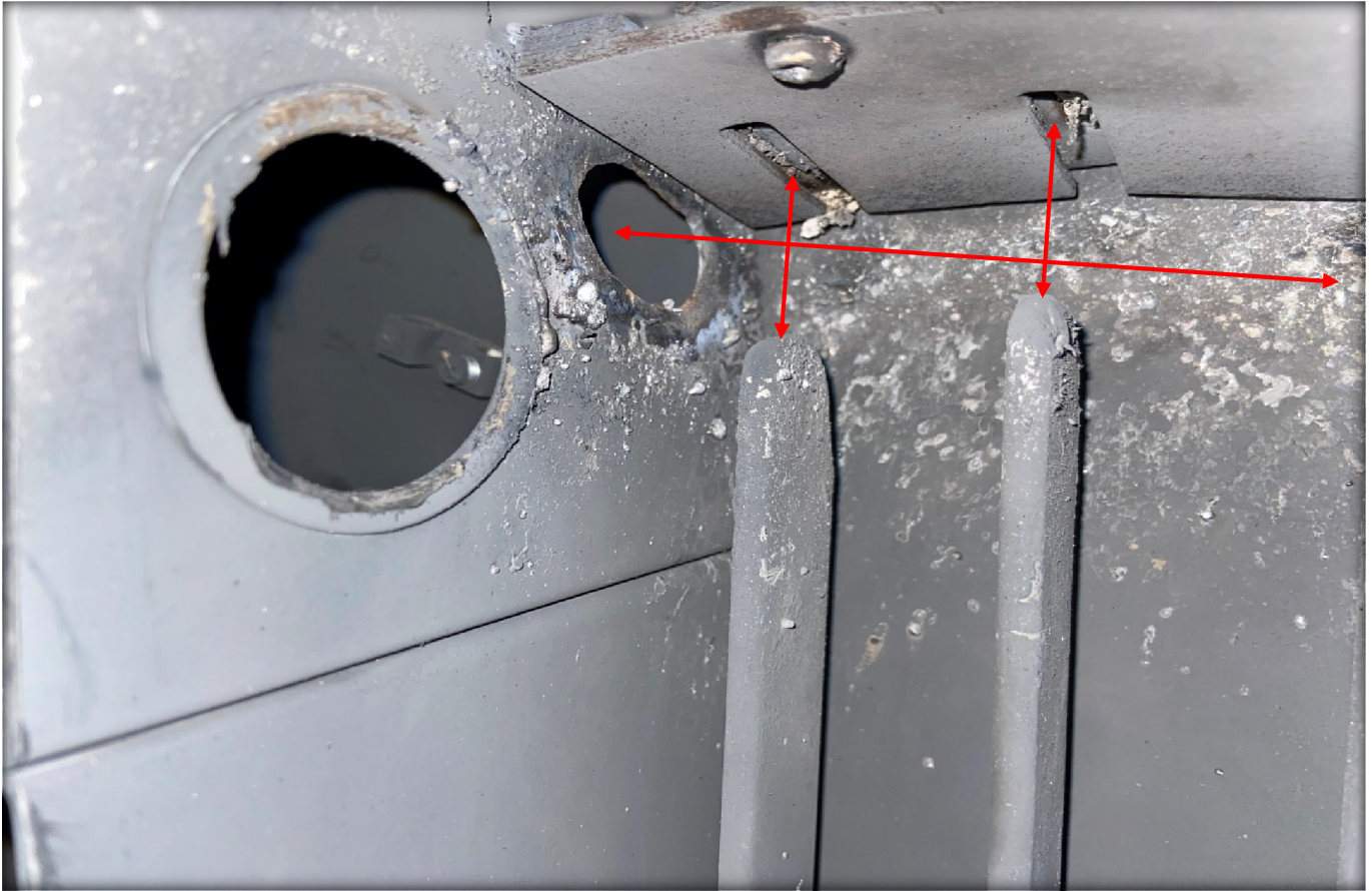
Figure 6 – Close up of bus bars and metal enclosure melted from the arc flash event.
